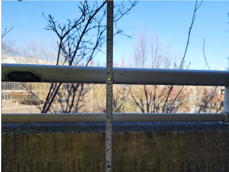
Level P5 garage pedestrian barrier less than 42 Inches in height
