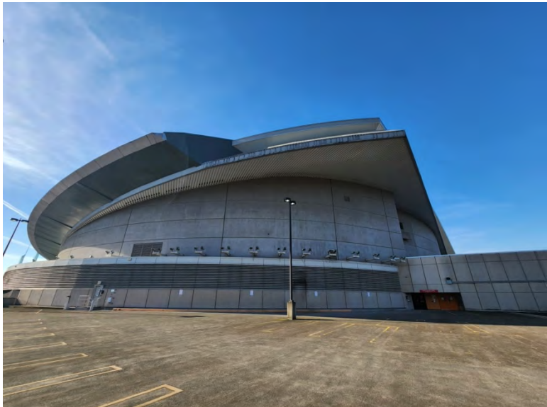
Dirt accumulation on precast and metal panels
