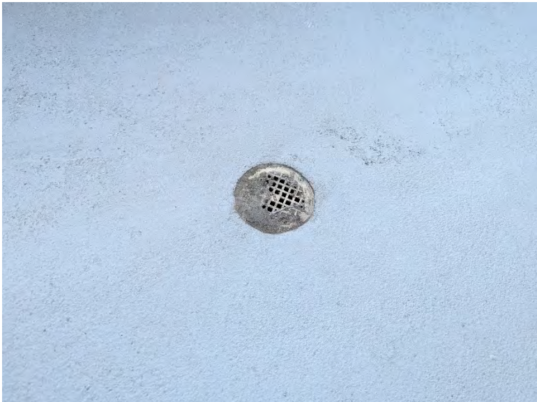
Club Level (Section 225) obstructed plaza annex floor drain
