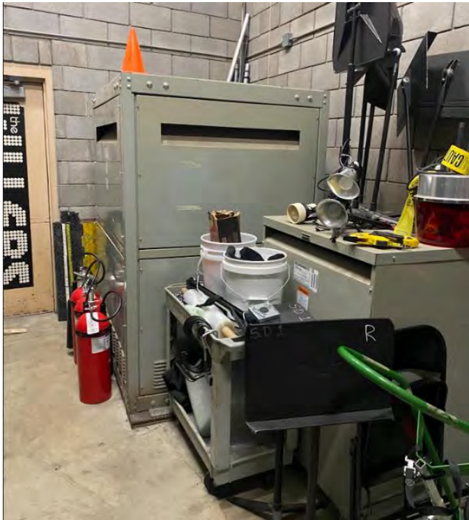
Storage violating NEC clearances
