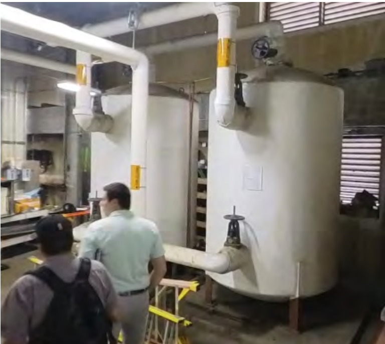
Domestic hot water storage tanks on club level
