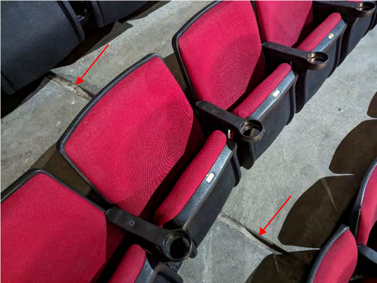
Seating bowl (Section 322) with locally failed joint sealant at seating row
