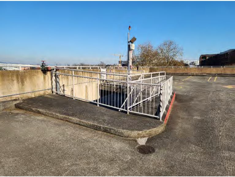
Level P7 missing stair vehicle barriers
