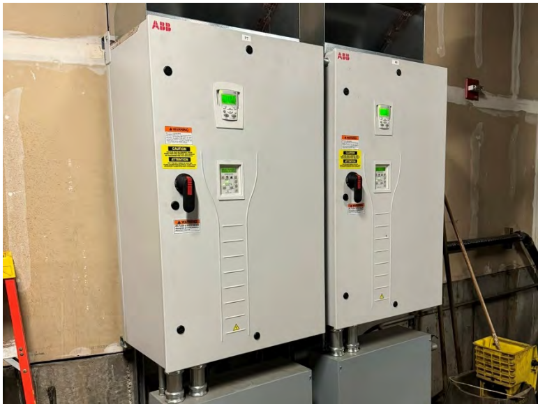
Secondary chilled water pump VFDs
