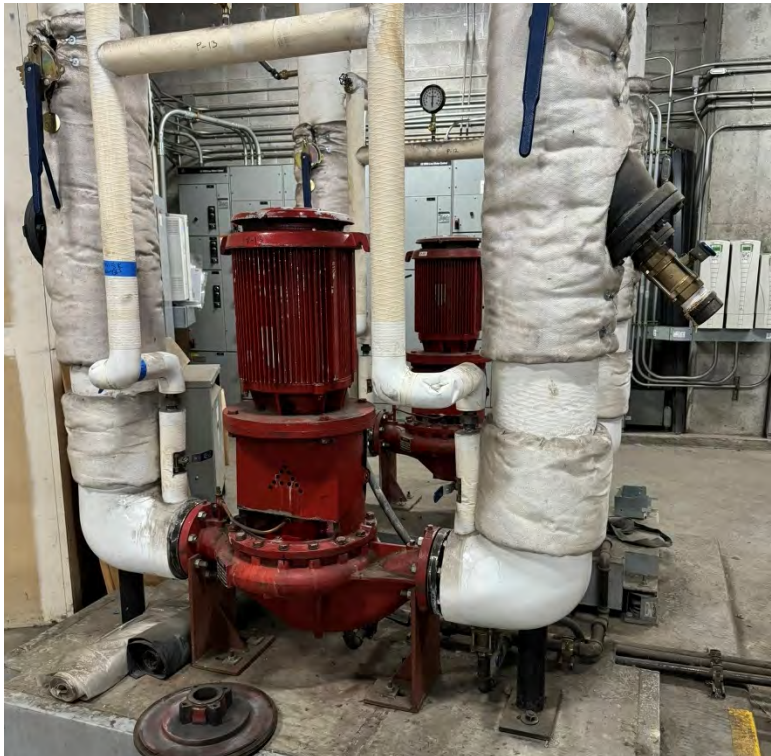
Heating hot water secondary pumps
