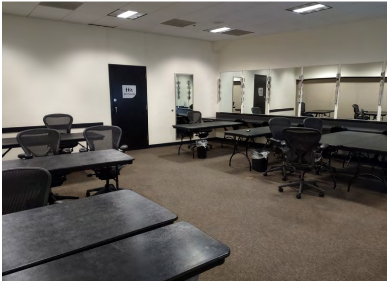
Star dressing rooms have older finishes on floor, walls & ceilings show signs of wear and tear
