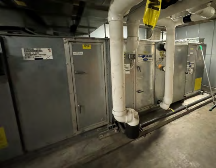
Support air handling unit
