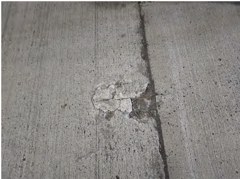
Level P1 spalled floor slab
