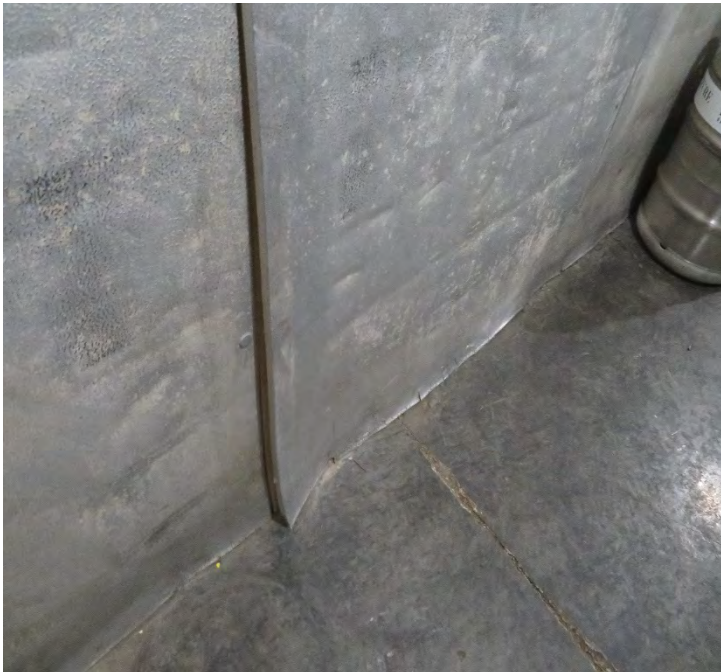
Damaged walls from beer kegs
