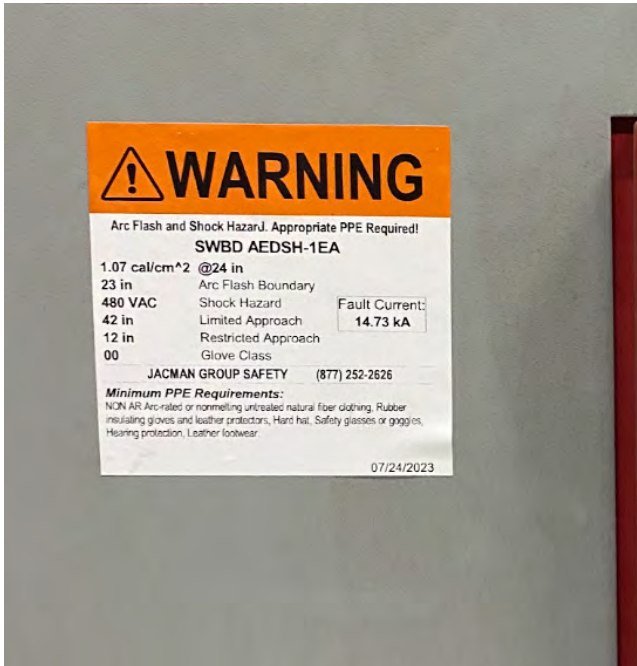
Typical arc flash label
