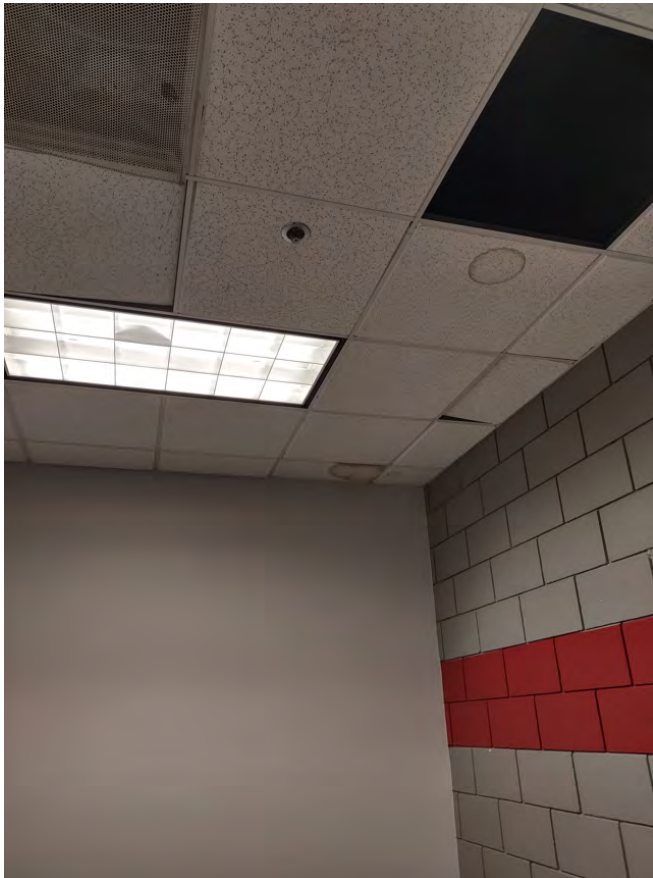
Water stain observed on ceiling tile in media workroom
