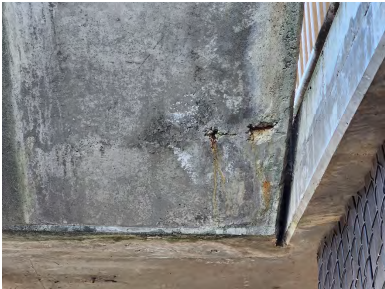
Level P4 overhead concrete spalling
