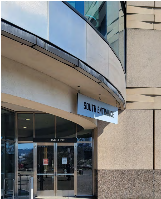
Dirt accumulation on metals and precast panels
