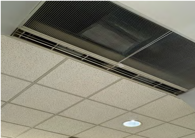
Air curtain at restroom
