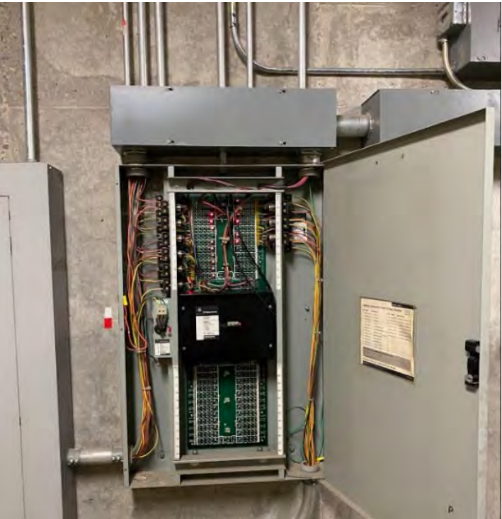
Typical lighting contactor cabinet
