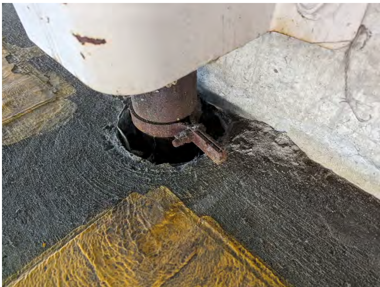
Level P6 unsealed pipe penetration
