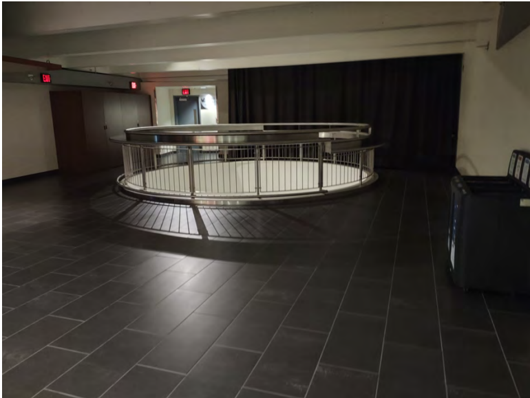
Concourse at Club Level tile flooring in fair condition
