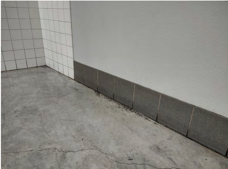
300 Level toilet rooms have original finishes with wall tile and base show signs of wear and tear
