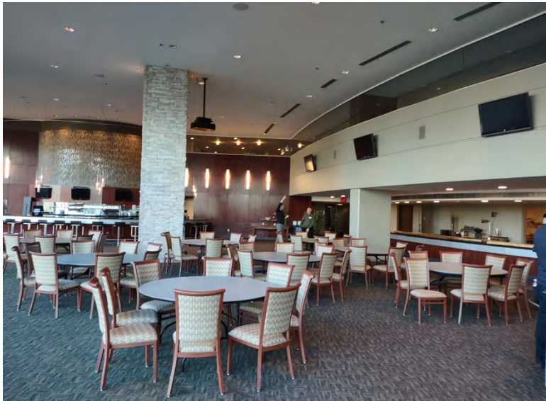
Lounge at club level carpet shows signs of wear and tear
