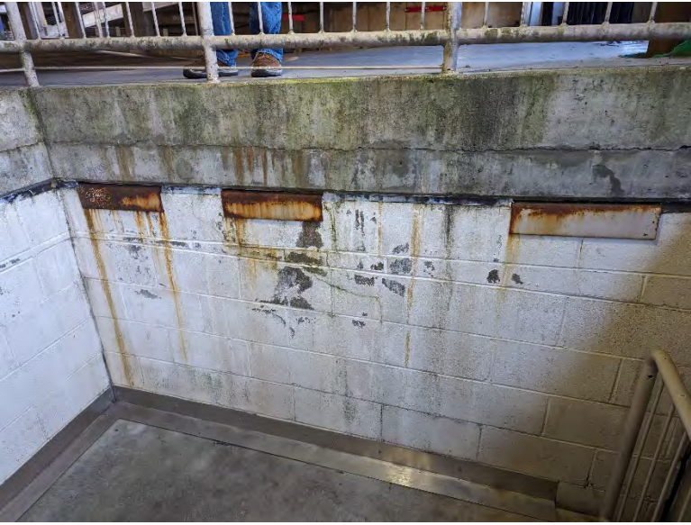
Level P4 cracked CMU wall
