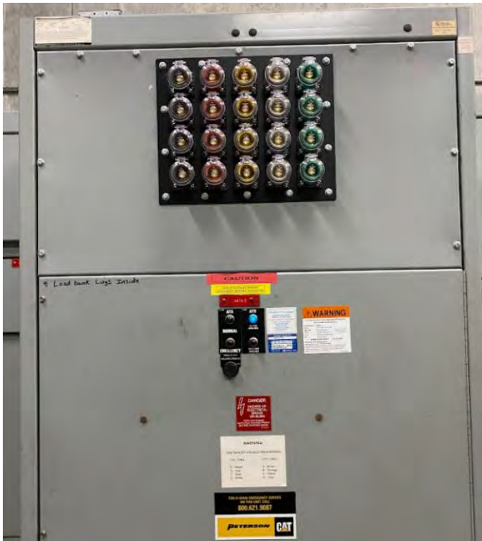
AATS-2 with load bank connections
