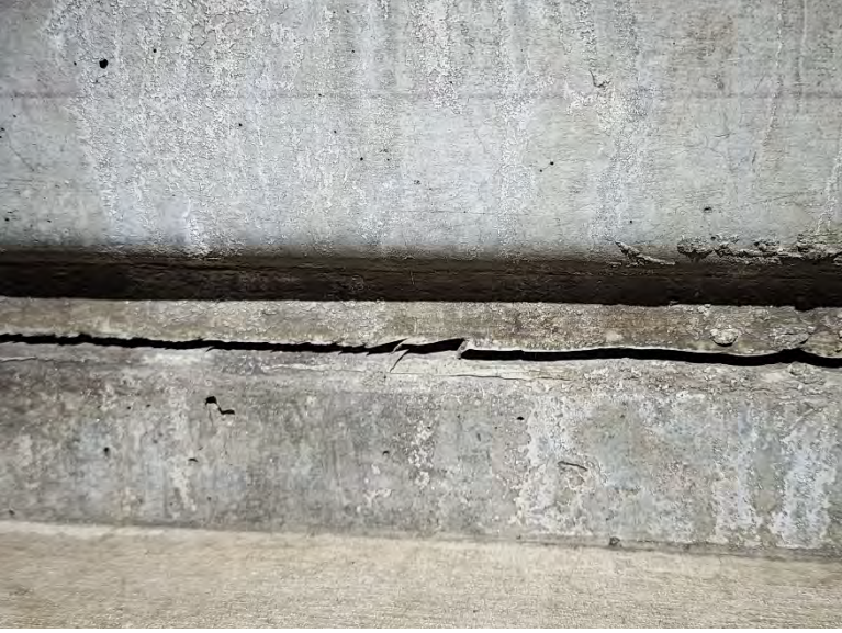
Seating bowl (Section 314) with locally failed joint sealant at stair riser
