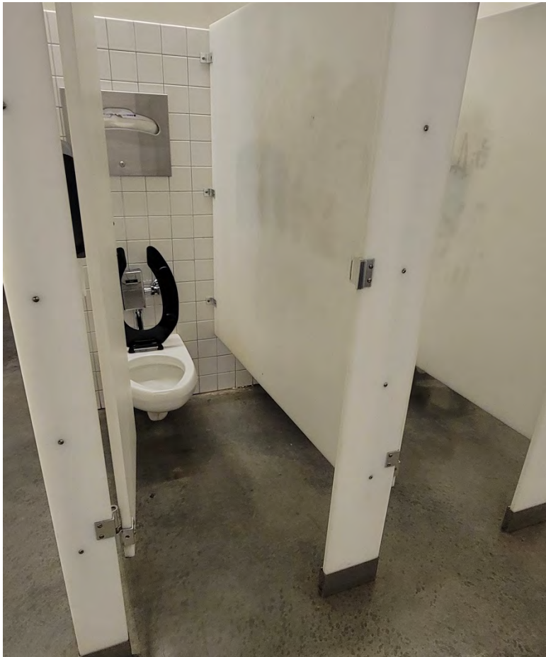
Toilet room partition material showing ghosting of prior graffiti cleaning
