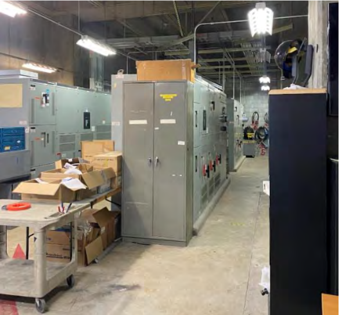
Main electrical room
