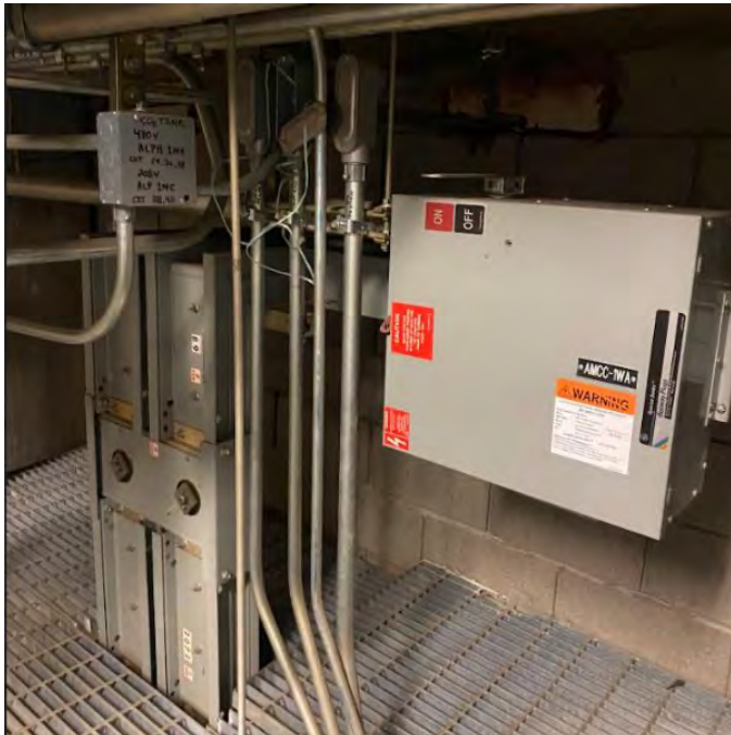
Bus duct riser
