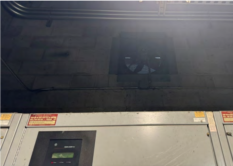
Ventilation fans in main electrical room
