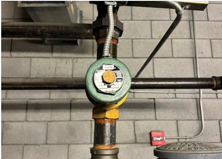
Pump in fuel storage room
