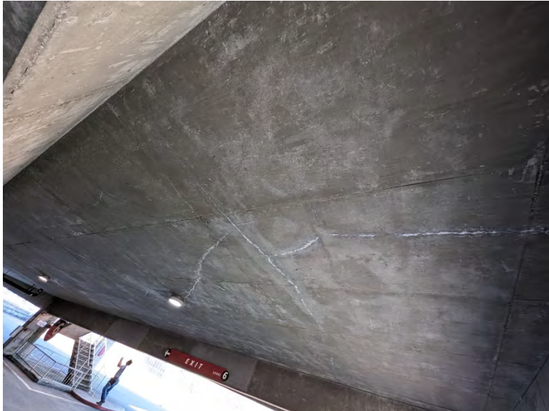
Level P6 soffit cracking and efflorescence
