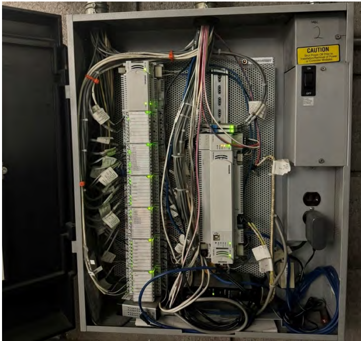
Building automation system control panel
