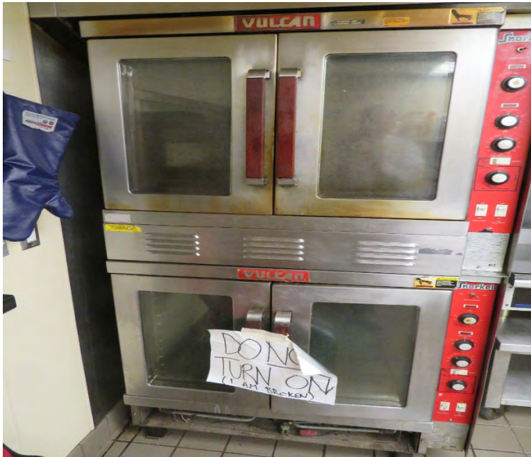
Signage on non-working equipment
