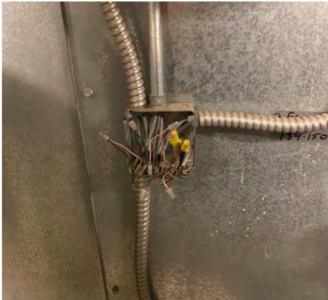
Example of exposed junction box
