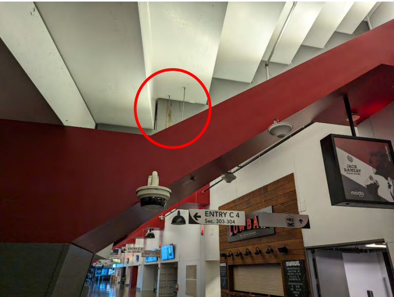
Upper concourse (Section 303) staining at cast-in-place raker
