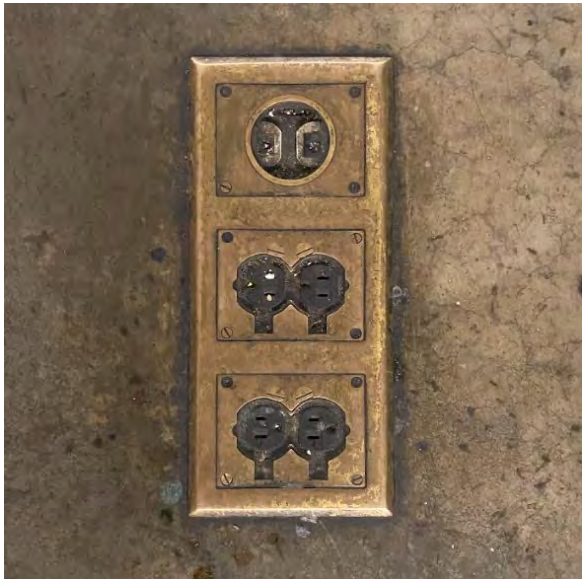
Damaged poke-thru receptacle on concourse
