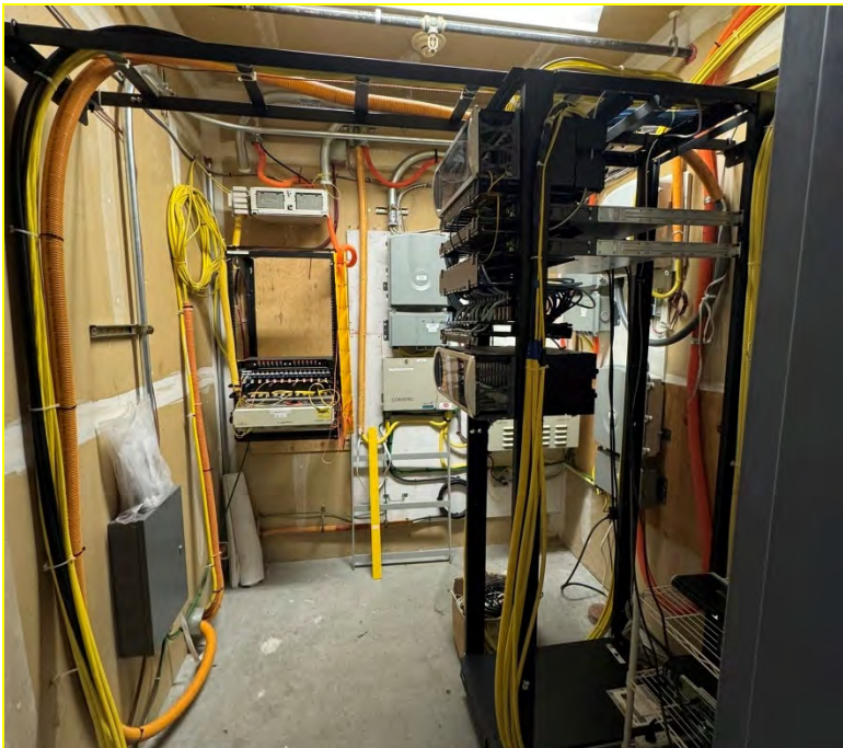
Catwalk level IT closet
