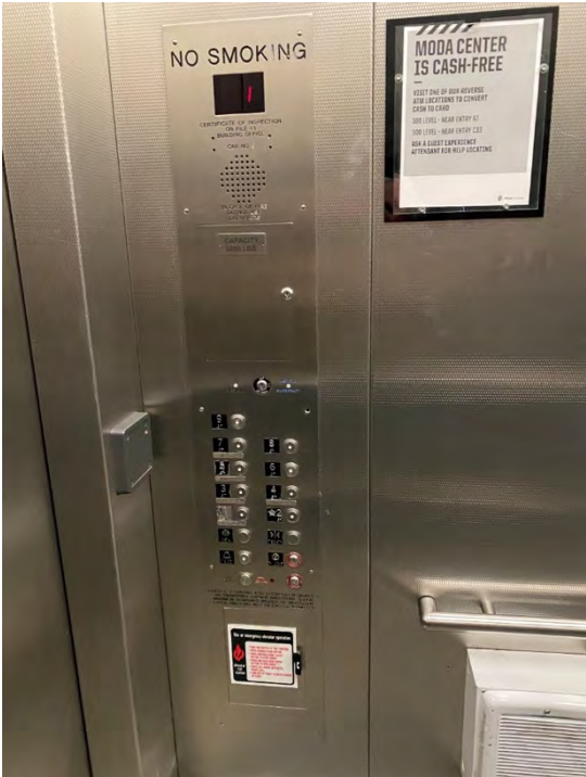
Elevator PE6 car operating panel showing Floor 9 button
