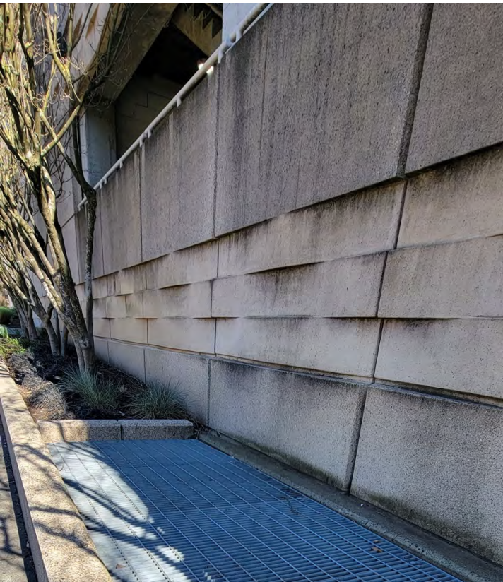
Dirt accumulation on precast panels
