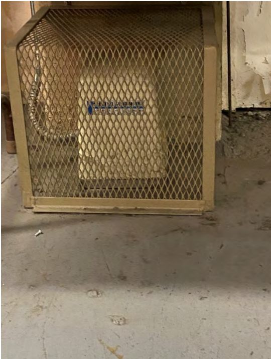
One seismic switch for all elevators in the Rose Quarter located in the Garden Garage machine room
