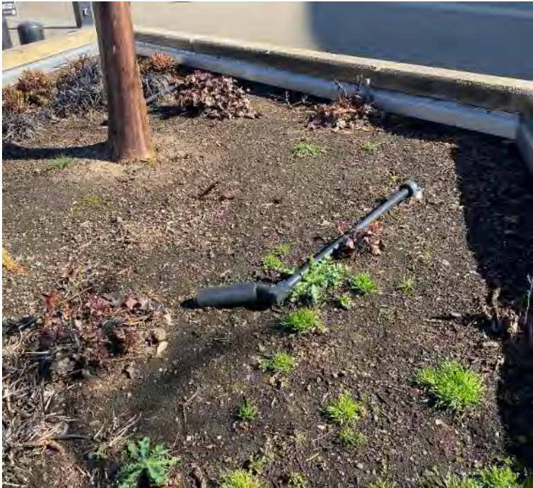
Vandalized garden bed fixture
