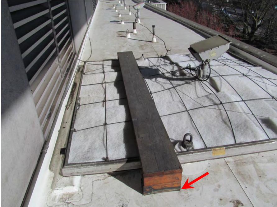
Wood plank, provided for foot traffic across a filter blanket, is installed directly on the (unprotected) roof membrane surface
