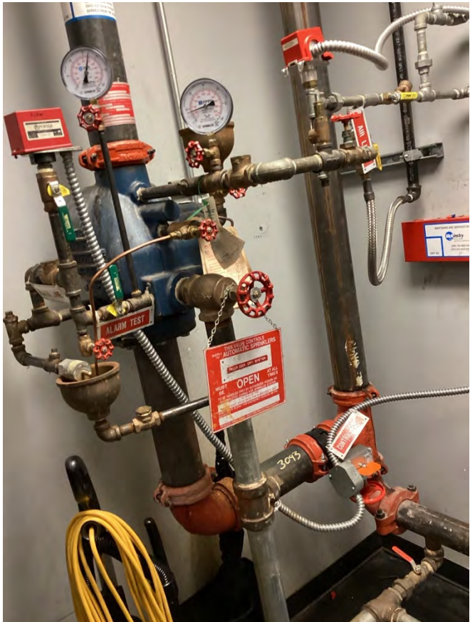
Dry sprinkler valve serving loading dock
