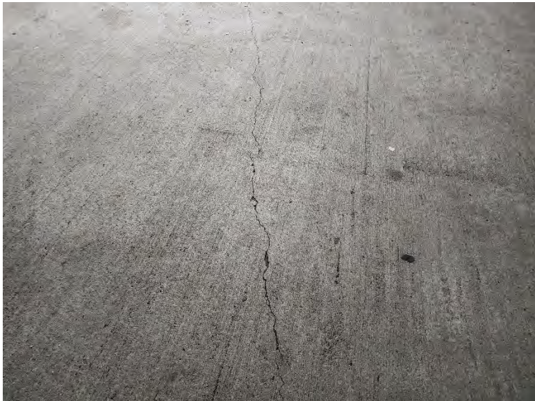
Level P2 below grade floor cracking
