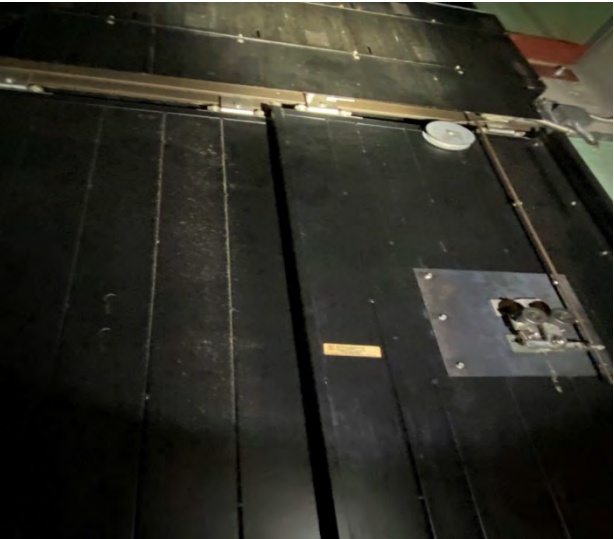
Typical hoistway door
