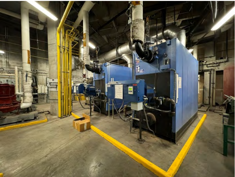
Boilers B-1 and B-2
