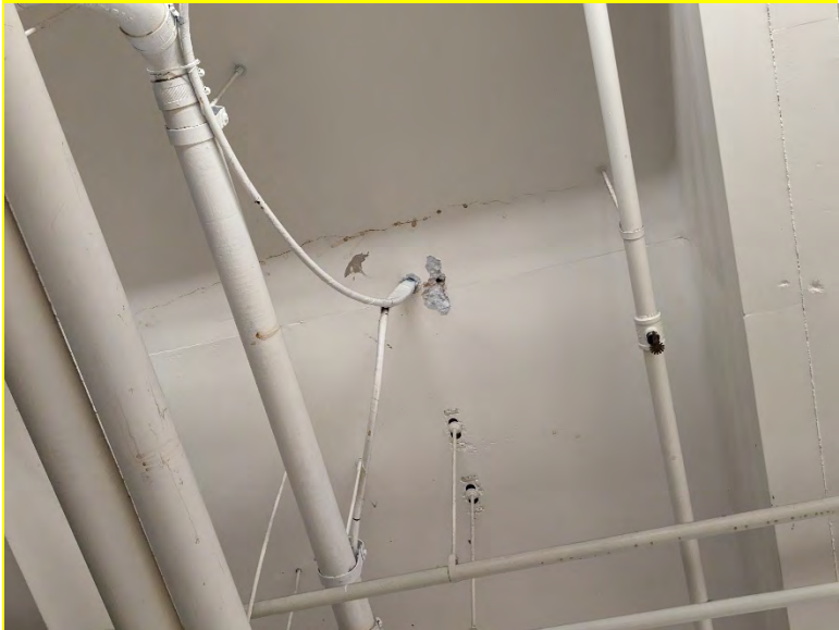
Main concourse (Section 114) concrete pan joist soffit spalls at previous anchor locations
