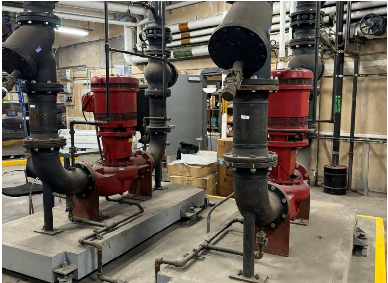
Heat recovery condenser water pumps
