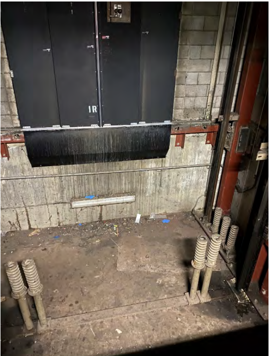
Pit of Elevator PE5 in need of cleaning
