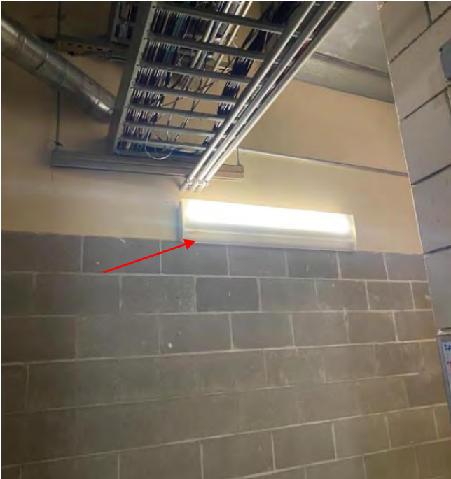
Burned out wall mounted fixture
