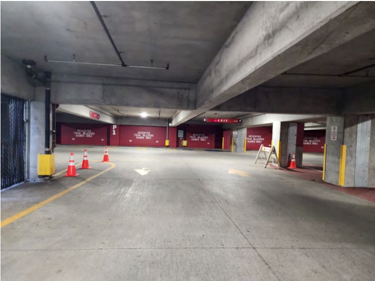
Wayfinding signage hidden with structural members
