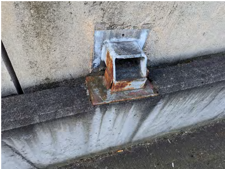
Level P7 corrosion at precast concrete façade panel connection
