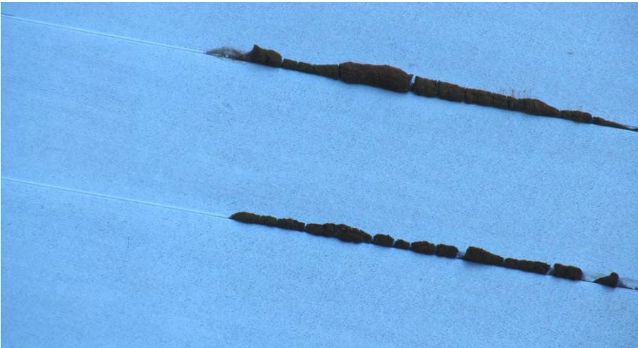
What appears to be mossy vegetation growing in seams of the mansard panels on the north elevation
