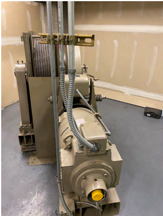
Montgomery geared traction elevator well maintained
