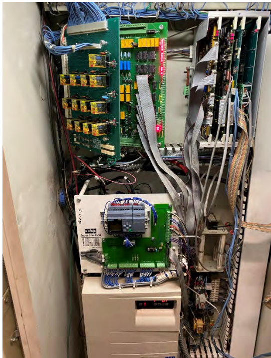
The elevator controller is in good condition
