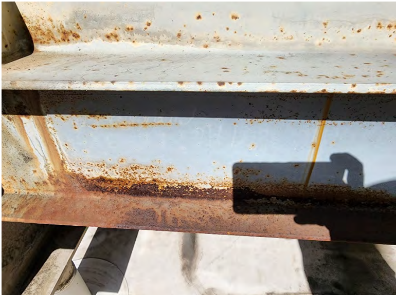
Mechanical level (Gridline R82-FF) corroded steel MEP framing beam
