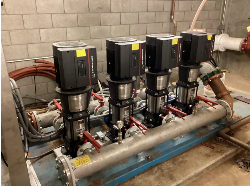
Quadraplex domestic water booster pump skid
