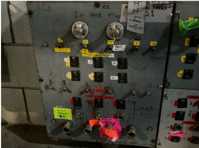
Player tunnel IO panel with temporary labeling
