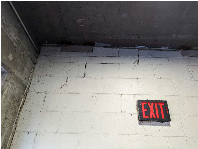
Level P4 cracked CMU wall
