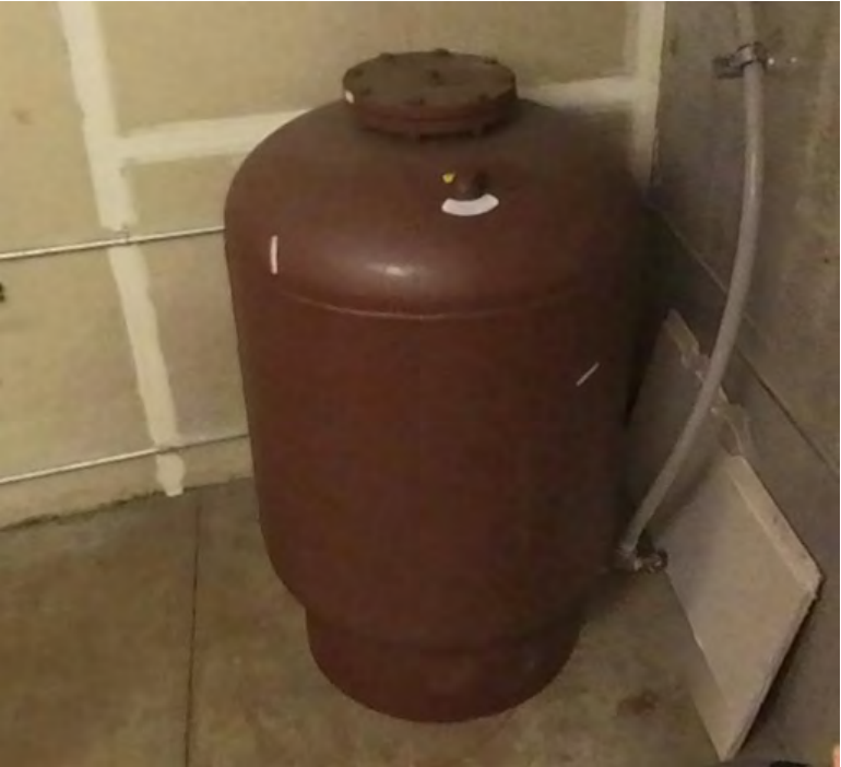
170 gallon hydropneumatic tank in fire pump room
