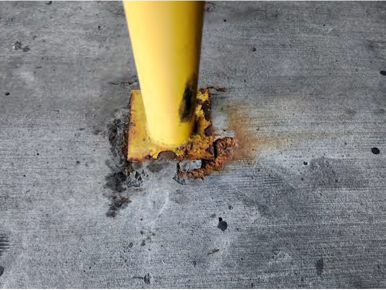
Level P4 corrosion at steel bollard base
