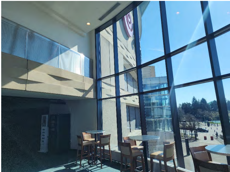
Club Level (Section 229) water Intrusion at fenestration
