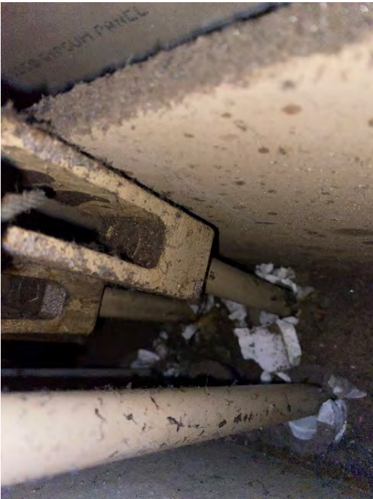
Disintegrating grommets in the counterweight
