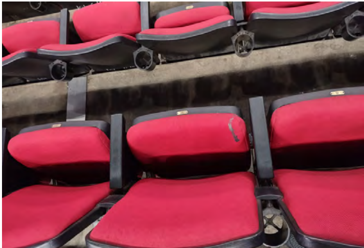
Stains on padded seating at lower deck
