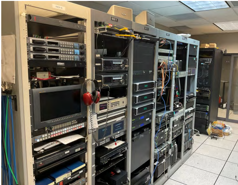
Production suite rack room – viewing row 2 of 2
