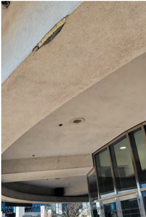
EIFS soffit damage
