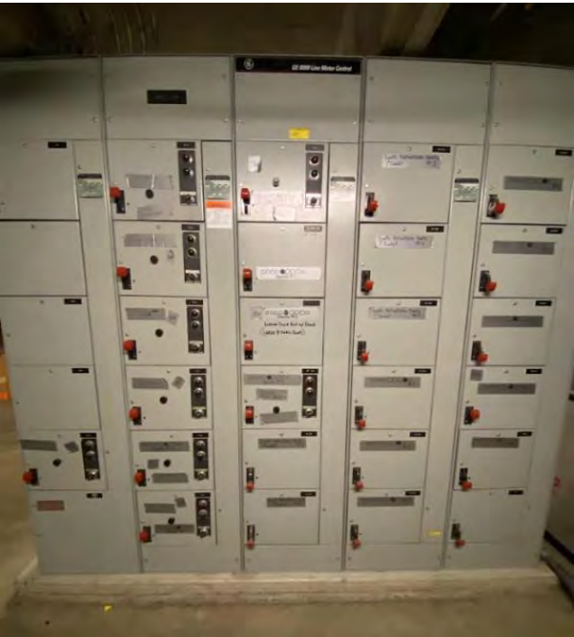
Typical motor control center
