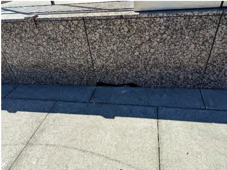
Façade (East façade) with spalled granite façade panel
