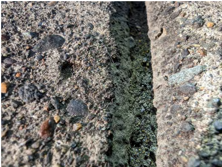
Level P7 floor slab construction joint without joint sealant
