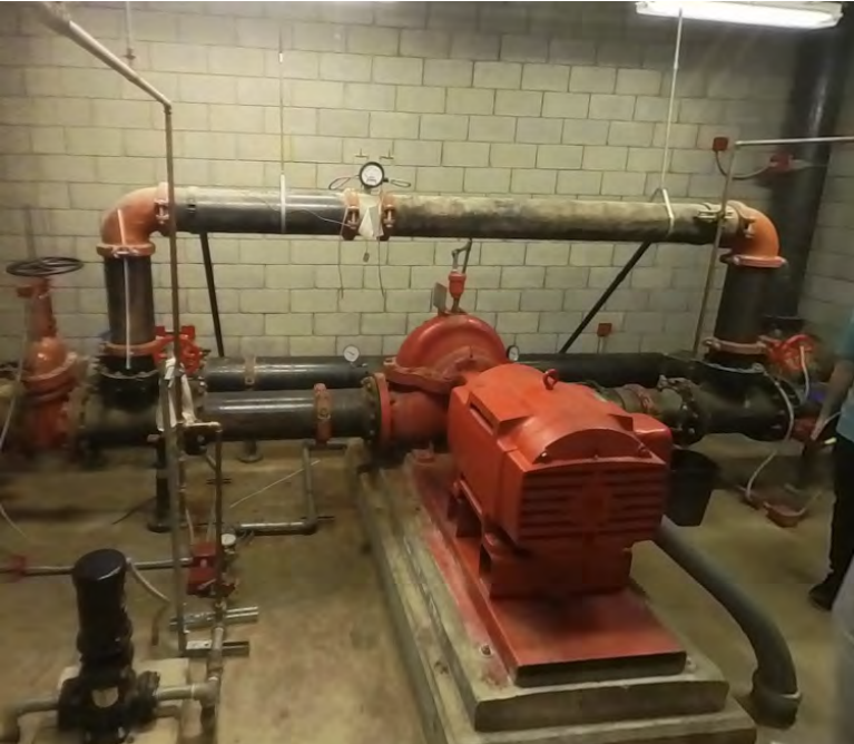
2500 GPM Peerless 8AEF17N 150 HP fire pump and jockey pump
