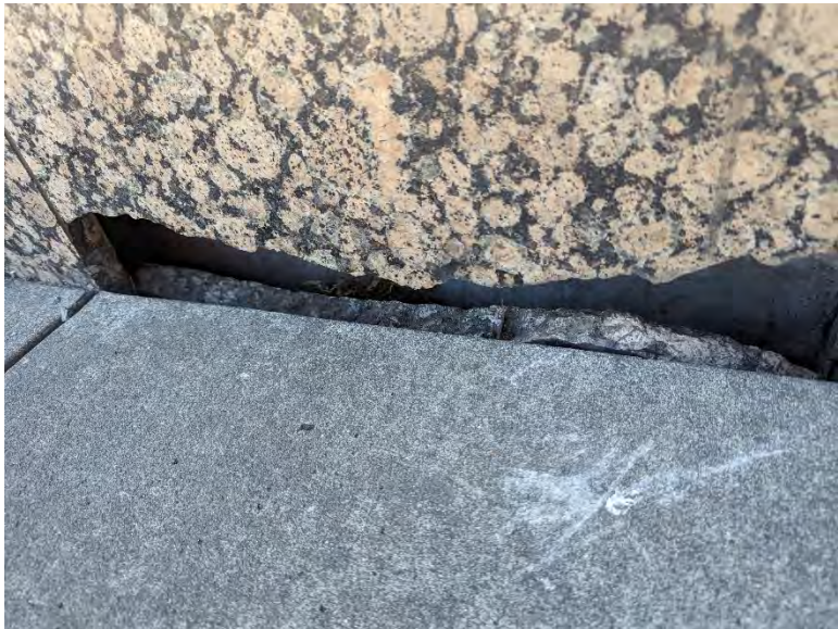
Façade (East Façade) spalled granite façade panel
