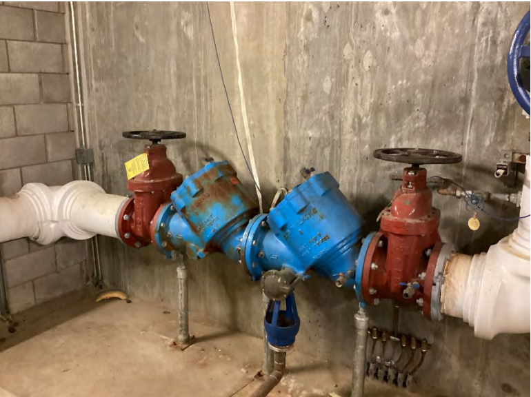
8" backflow preventer at water entry
