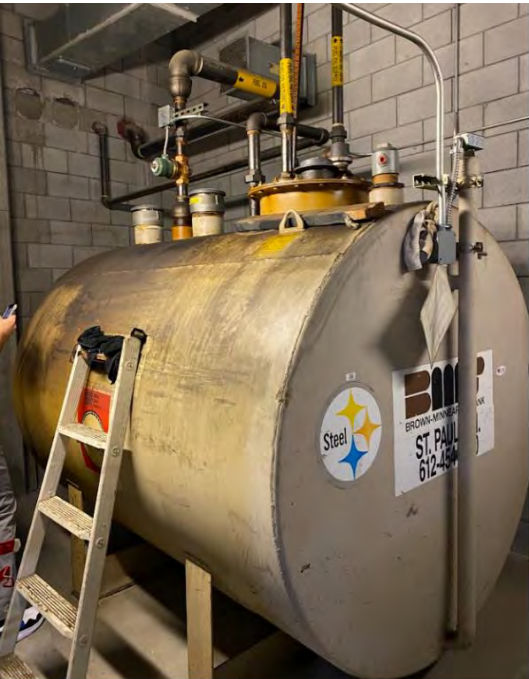
Diesel fuel tank
