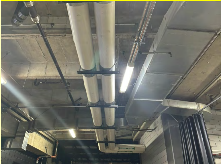
Abandoned ice floor brine piping
