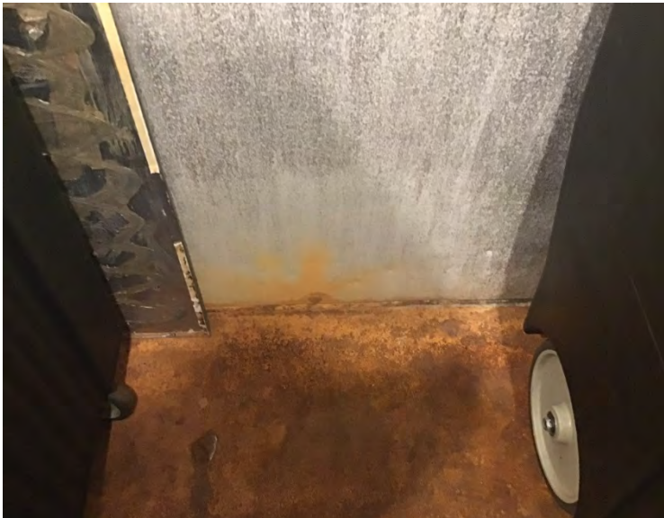
Rusting interior cooler floors
