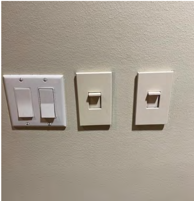
Local control switches and dimmers
