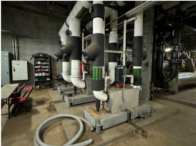
Chilled water primary pumps
