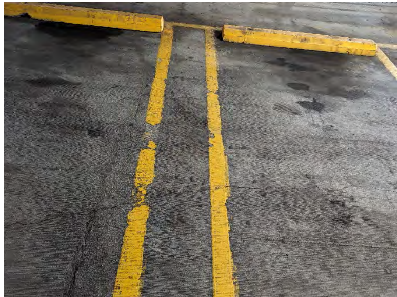
Level P4 ground level floor cracking
