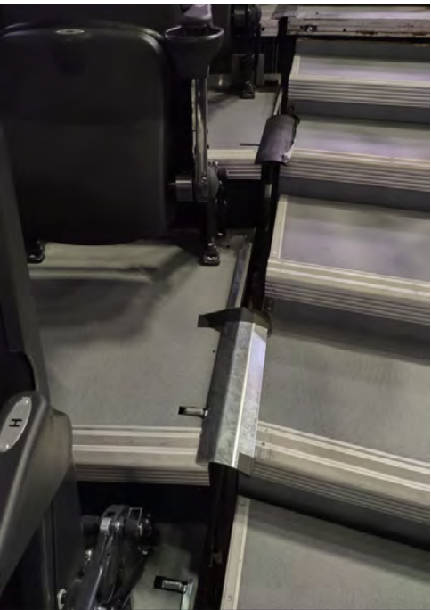
Aluminum closure plate at seating tread held in place with duct tape; this condition could become potential tripping hazard
