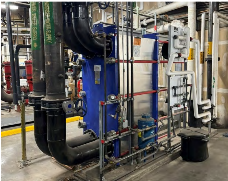
Heat recovery heat exchanger
