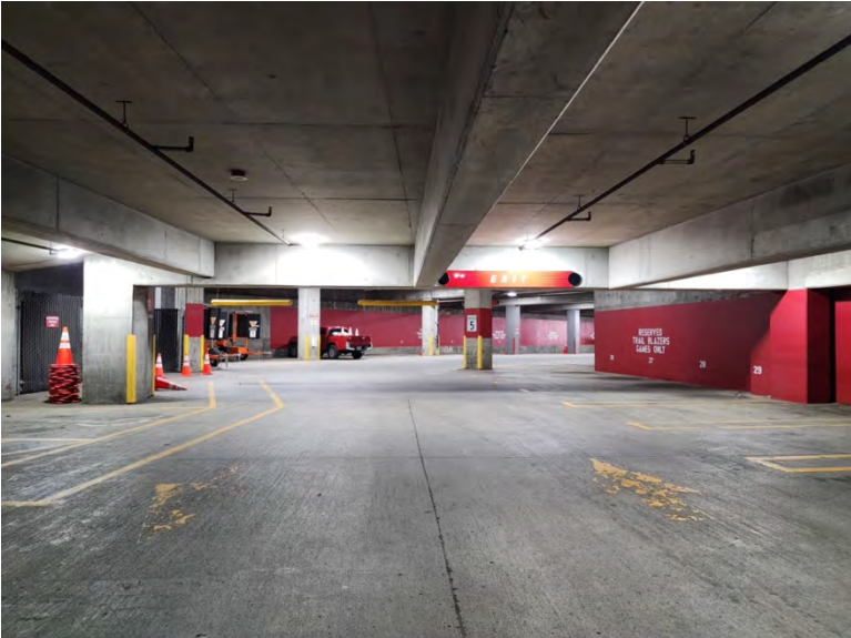
Light fixture imparting glare on wayfinding signage
