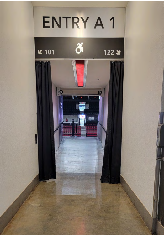
Polished concrete finish staining adjacent to walls
