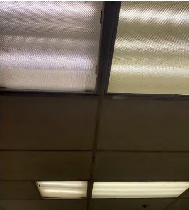
Aged fixtures in kitchen
