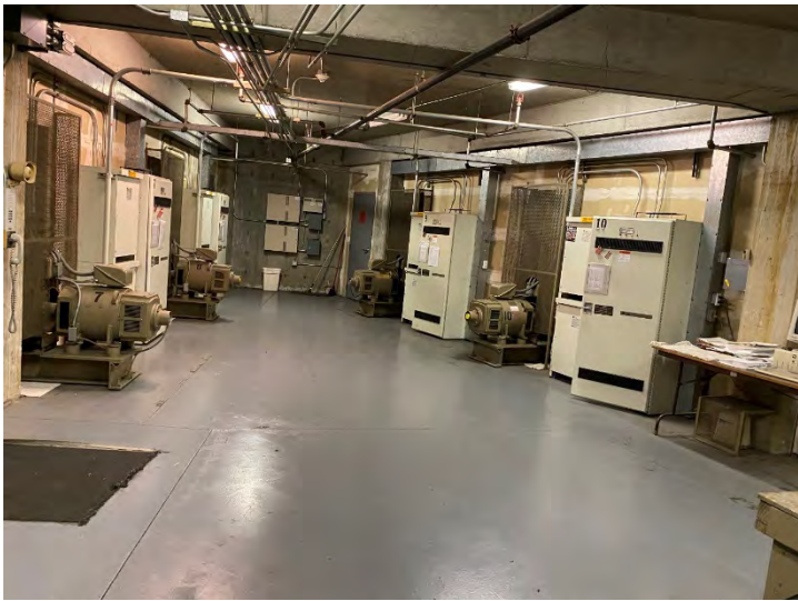
The machine room is clean and well organized with a seismic switch located in the Garden Garage machine room
