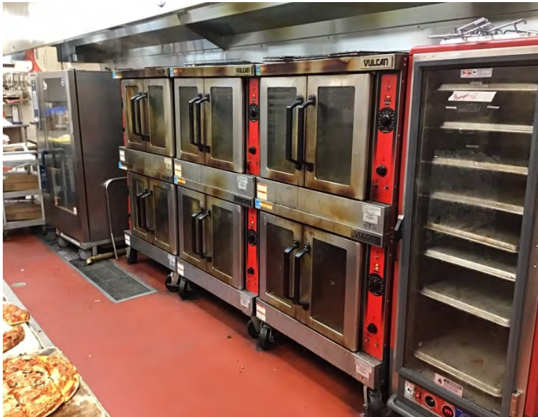
A bank of older convection ovens
