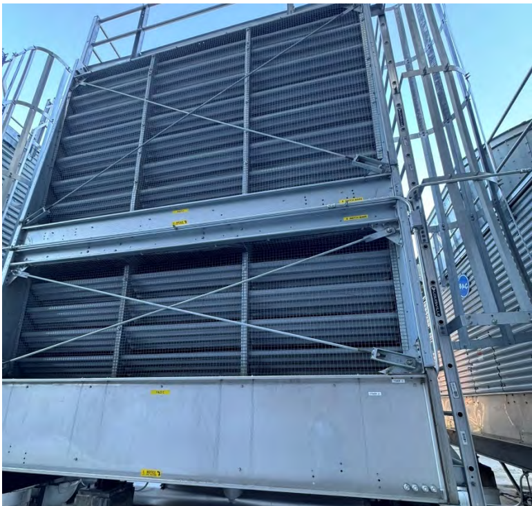
Chilled water system cooling tower
