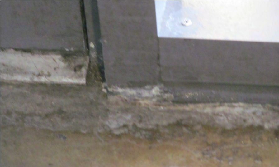
Moisture stains and damage along the base of storefront and entry door near northwest corner of terrace Roof Area 22
