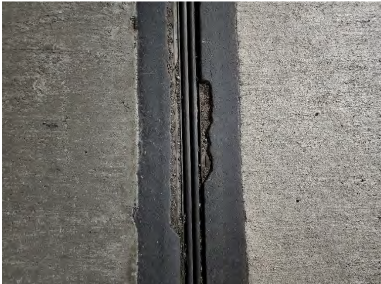
Level P2 compression seal expansion joint with damaged winged headers
