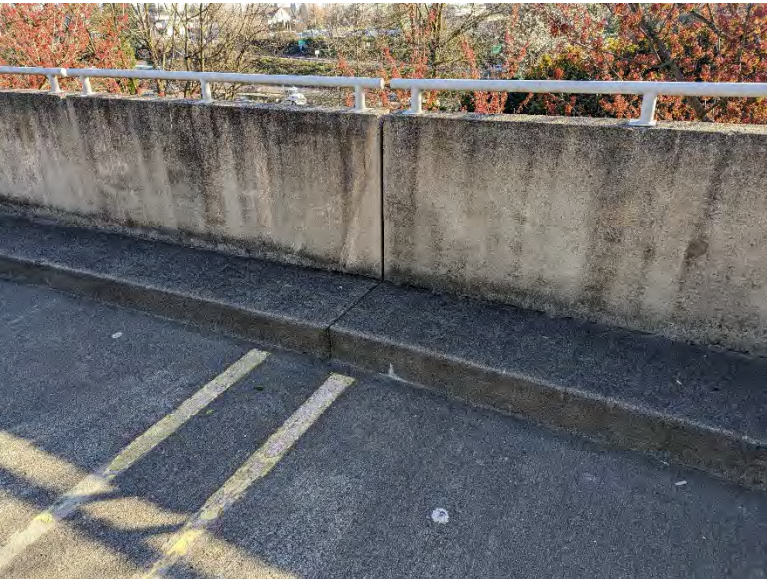
Level P7 perimeter walls and curbs without cove sealant
