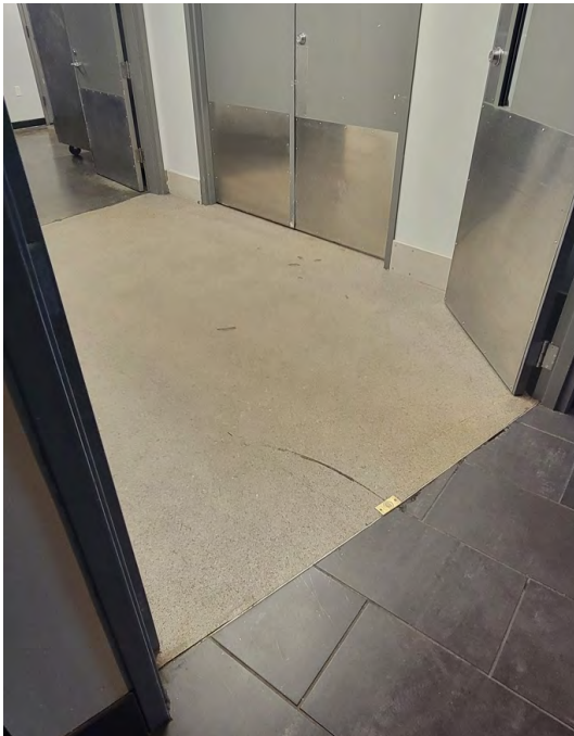
Club Level tile chipping and flooring wear
