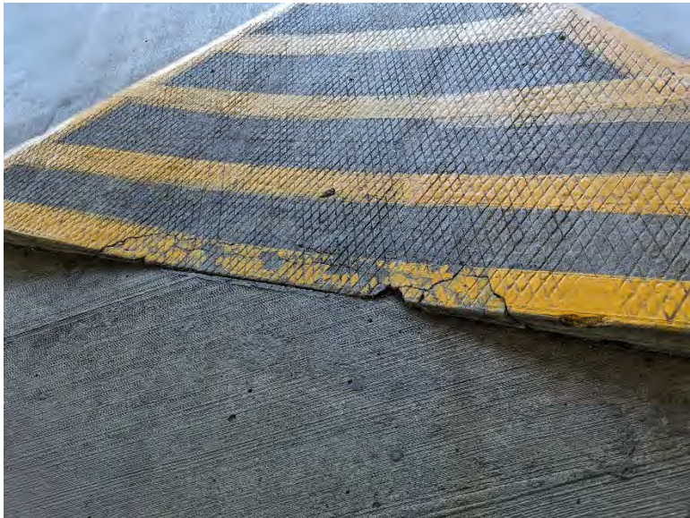
Level P4 cracked curb near the stairwell
