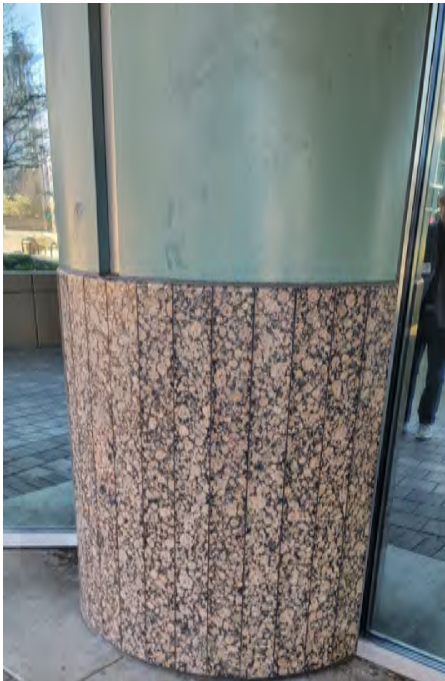
Metal column wrap baked on finish is oxidizing allowing handprints to easily mark finish appearance
