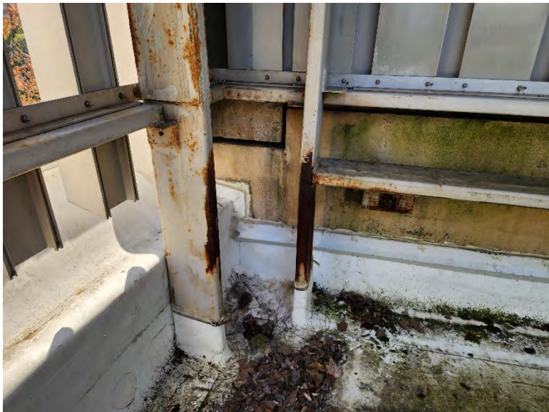
Mechanical level (Gridline R82-FF) corroded steel panels
