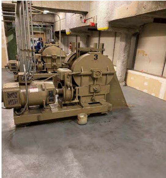
Elevator machine room for the Elevators PE2 and PE3 group
