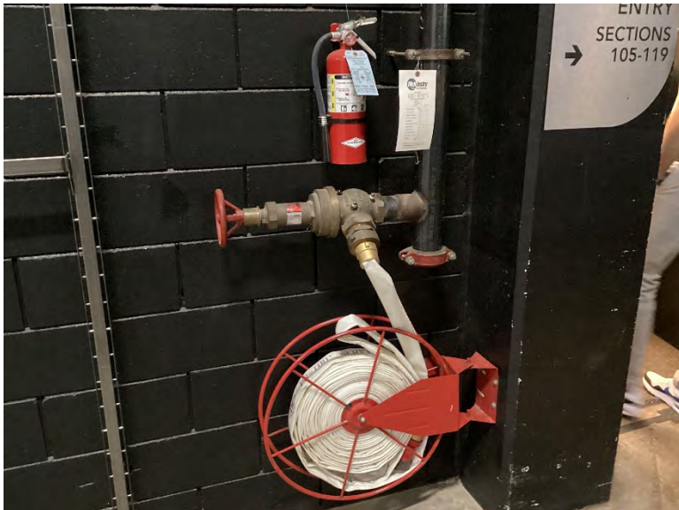
Typical fire hose reel on event level
