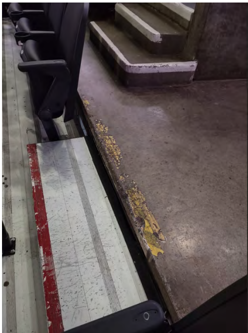
At Section 116 the gap between concrete and aluminum aisle step; this condition could become potential tripping hazard
