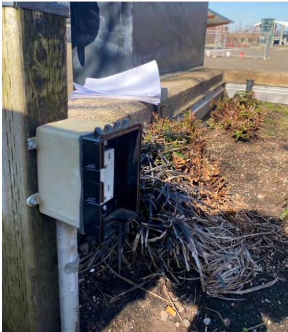
Missing weatherproof receptacle cover
