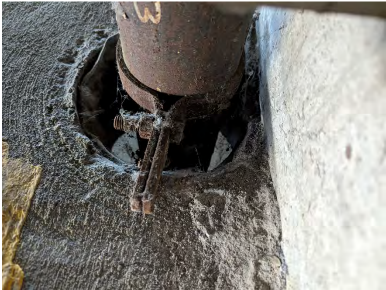
Level P6 unsealed pipe penetration
