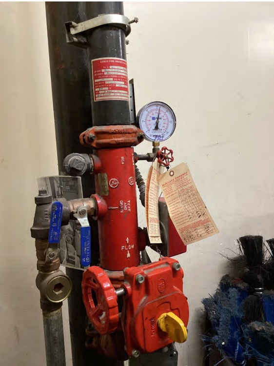
Typical wet zone control valve
