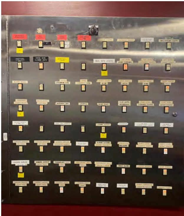
Wall mounted lighting control station
