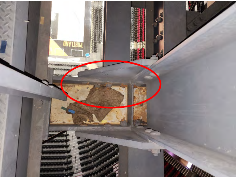
Catwalk level (Gridline R7) corroded steel framing bolt connection
