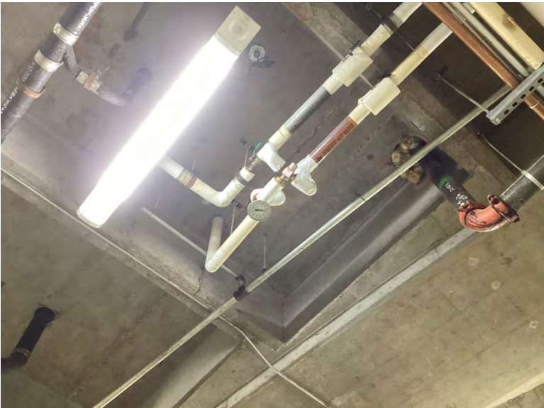
Typical point of use tempering valve in the ceiling of event level serving fixtures above
