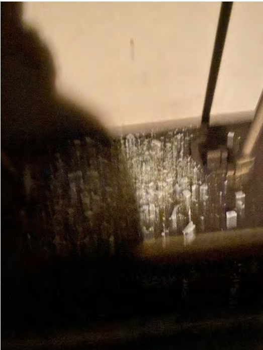
Disintegrating grommet material on the top of the counterweight
