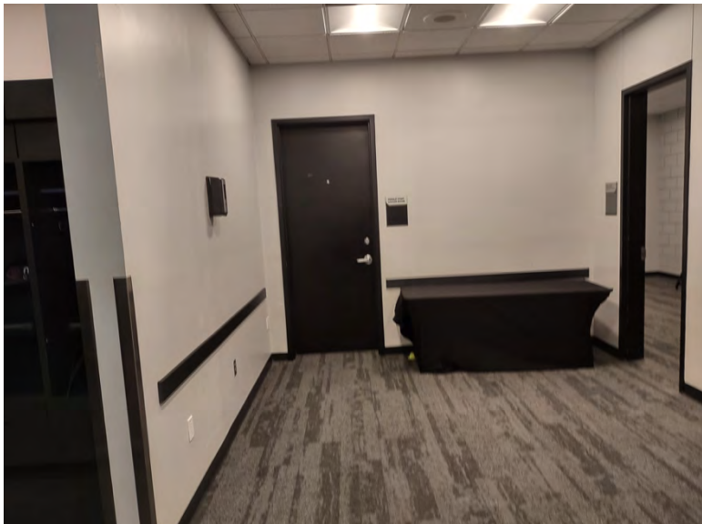
Auxiliary locker room architectural finishes on floor, walls, and ceilings show signs of wear and tear
