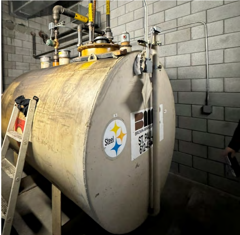
Fuel storage tank
