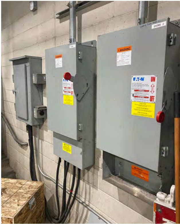
Additional 200A truck dock disconnects
