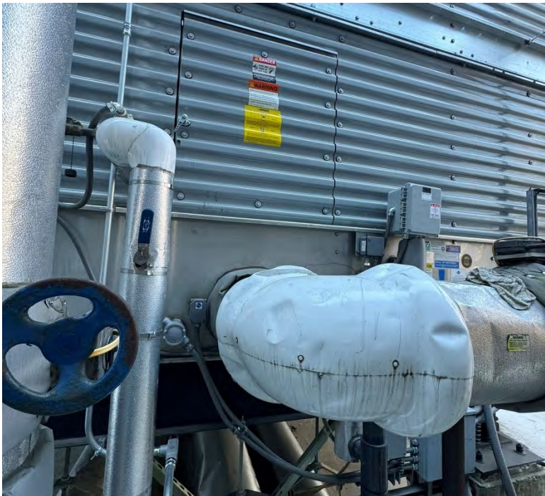
Cooling tower access
