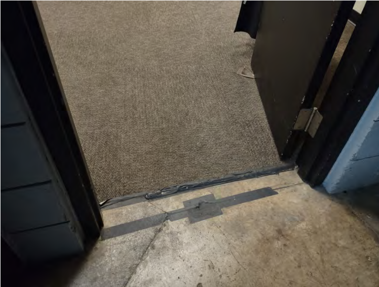
Door threshold at star room is worn out and needs repair/replacement to avoid potential tripping hazards
