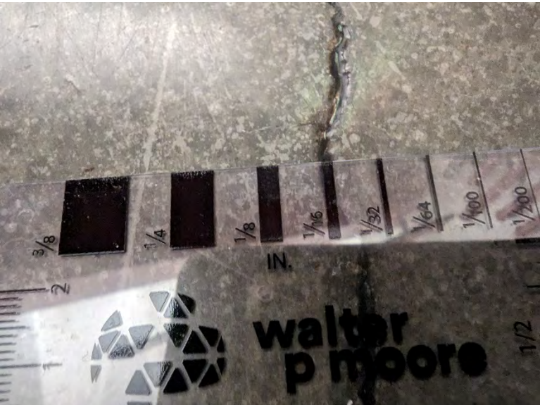
Upper concourse (Section 310) concrete topping slab cracking measured to be 1/16" wide
