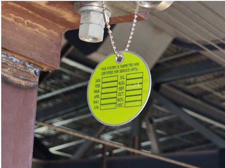
Catwalk level post installed fall protection system due for inspection in September 2024
