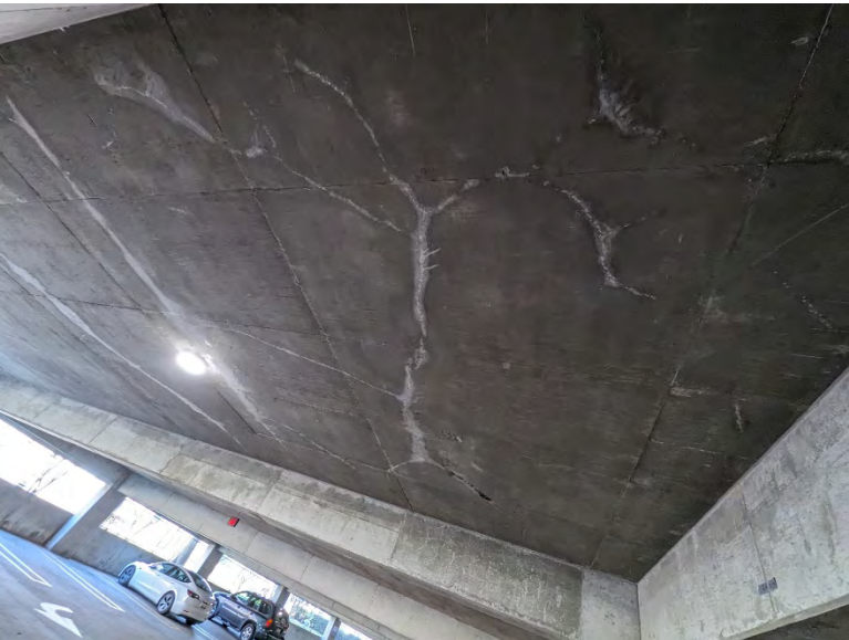
Level P6 soffit cracking and efflorescence below the helicopter pad
