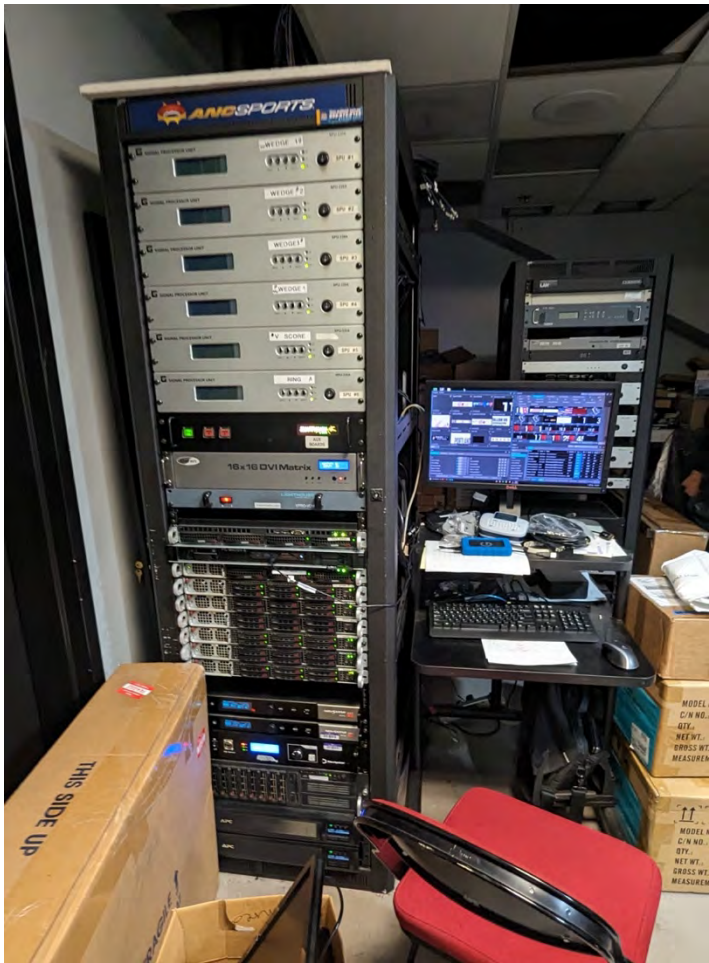
Existing LED processing and scoring system room
