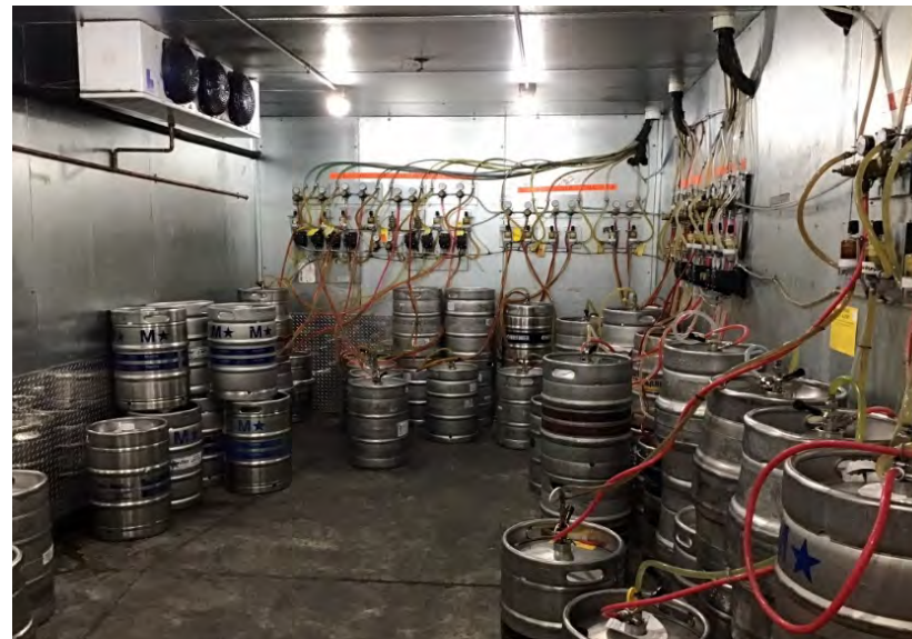
Draft beer walk-in cooler distribution
