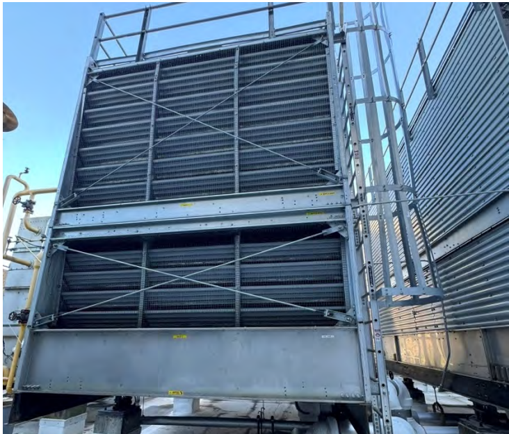
Heat recovery cooling tower
