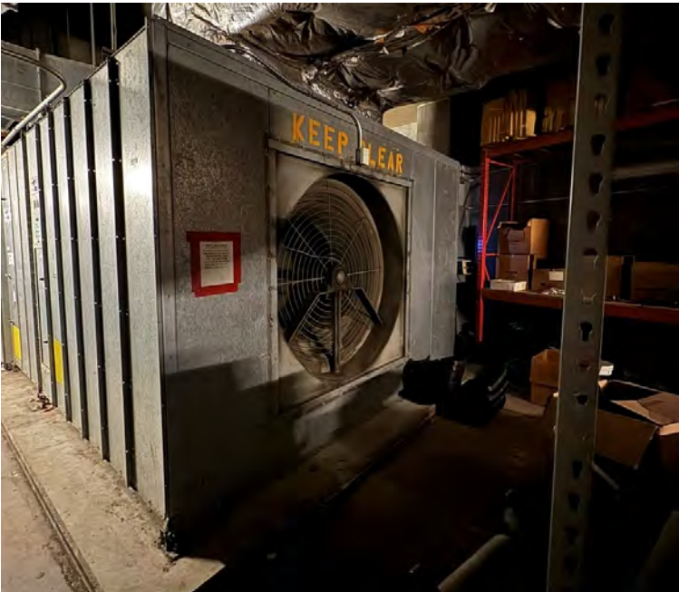
Support AHU open return
