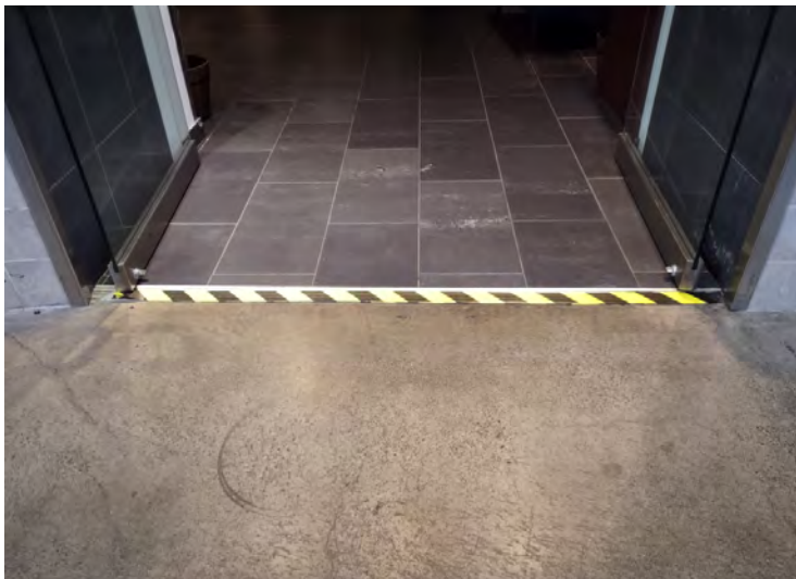
Floor transition at entry to Courtside Club needs repair/replacement to avoid potential tripping hazards or any accessibility issues
