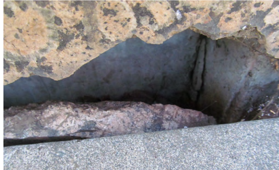
A piece of stone veneer is broken from a panel at/below grade, leaving an open gap
