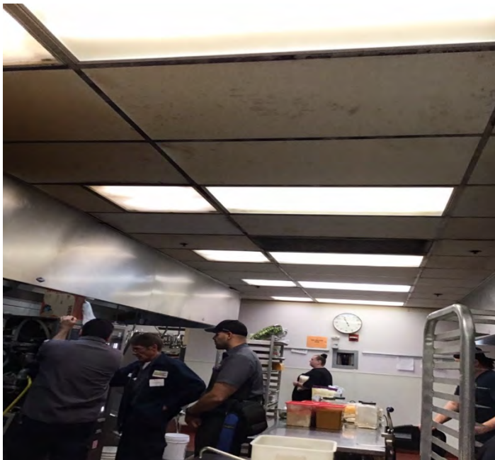
Kitchen ceiling tiles discolored
