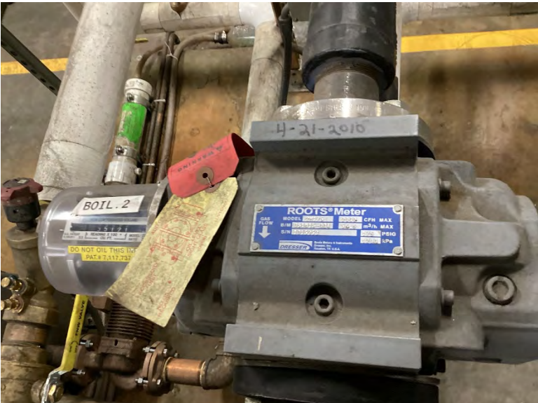
1 of 2 natural gas meters serving the domestic hot water boilers
