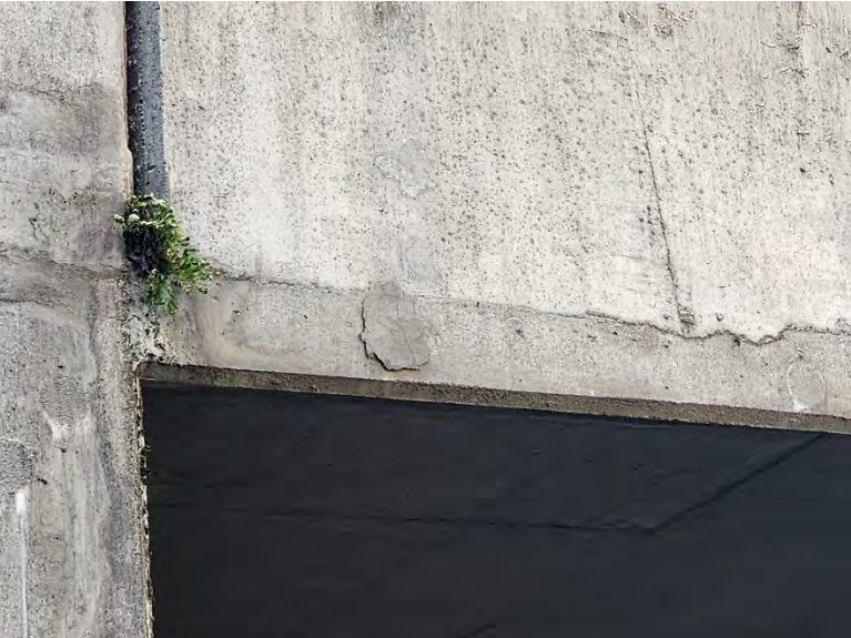
Level P6 post-tensioned tendon grout pocket delamination at the slab edge
