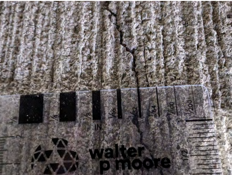
Level P4 ground level floor cracking measure to be approximately 1/32" wide
