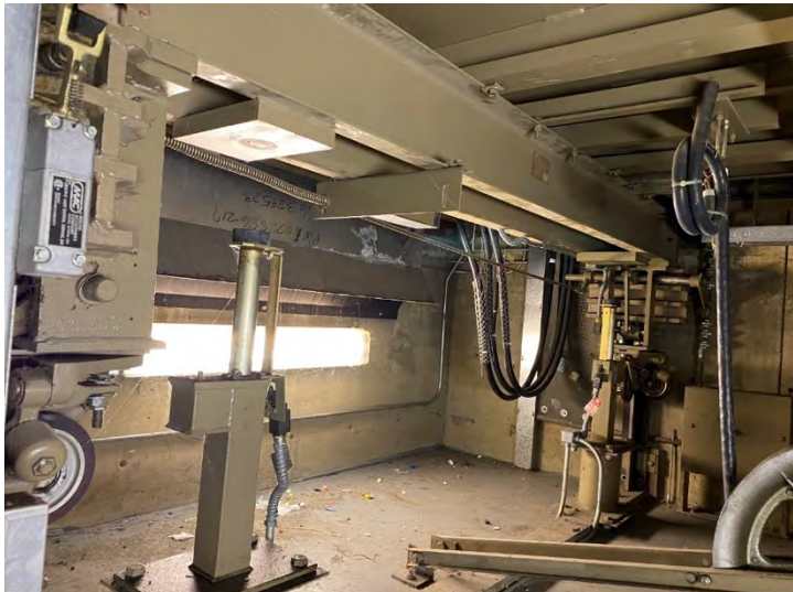
Underside of car is clean, well serviced with buffer tags attached per code
