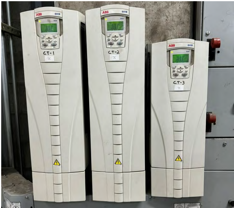
Cooling tower VFDs
