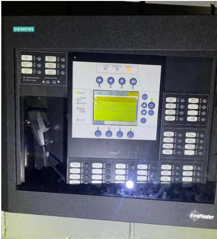
Siemens fire alarm cabinet with trouble message
