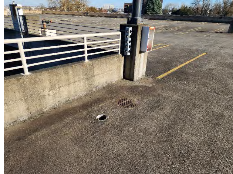
Level P7 slab penetration trip hazard
