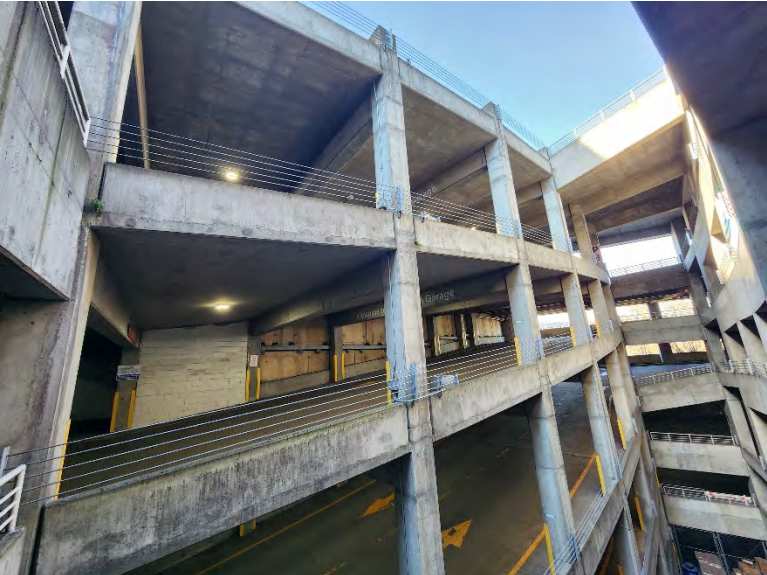
Level P5 post-tensioned tendon grout pocket delamination at the slab edge
