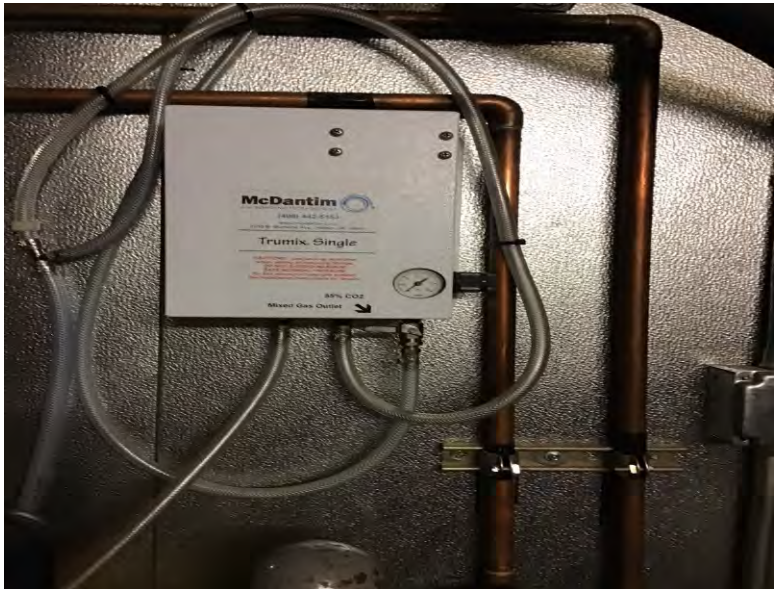
Individual Nitrogen blenders are in each cooler
