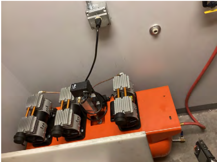
Air compressor serving dry sprinkler valve recently replaced
