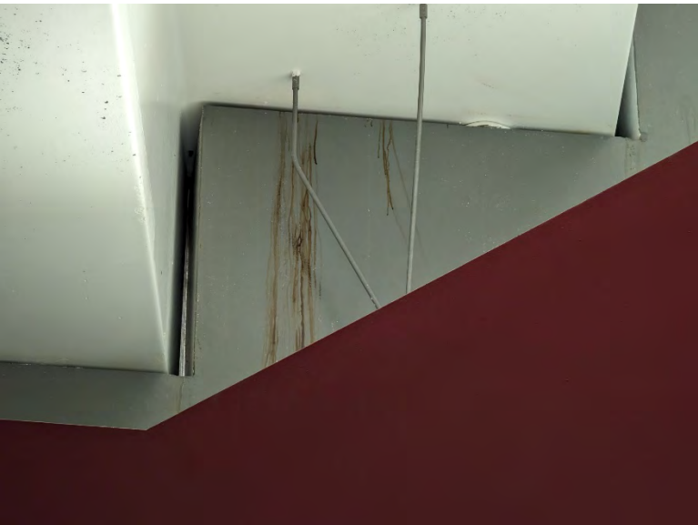
Upper concourse (Section 303) staining at cast-in-place raker
