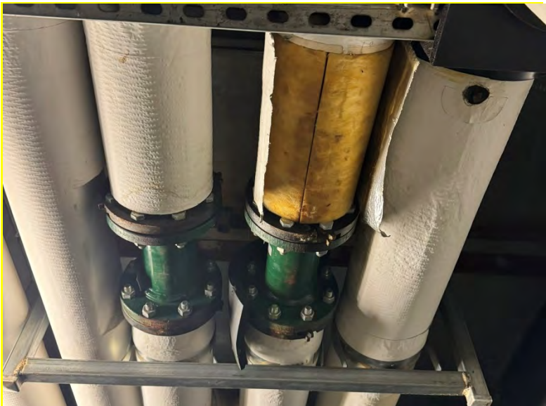
Damaged pipe insulation
