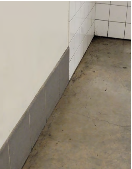
Polished concrete finish staining adjacent to walls
