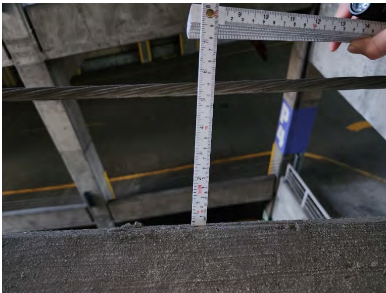
Level P5 garage pedestrian barrier gap greater than five Inches
