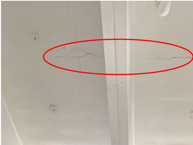
Main concourse (Section 121) concrete pan joist soffit cracking
