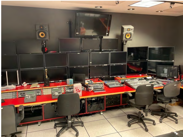
“Low Post” production control room main bench
