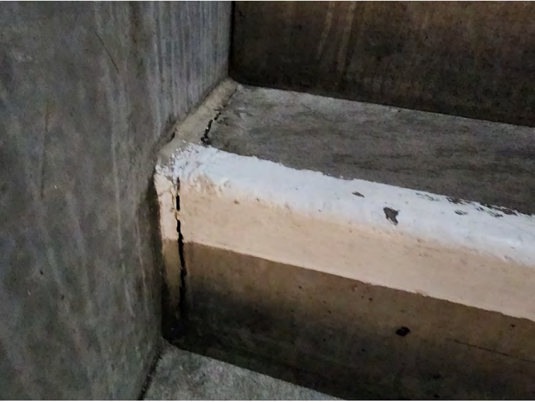
Seating bowl (Section 326) with locally failed cove joint sealant at stairs
