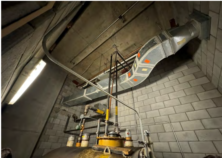
Ventilation fans in fuel storage room
