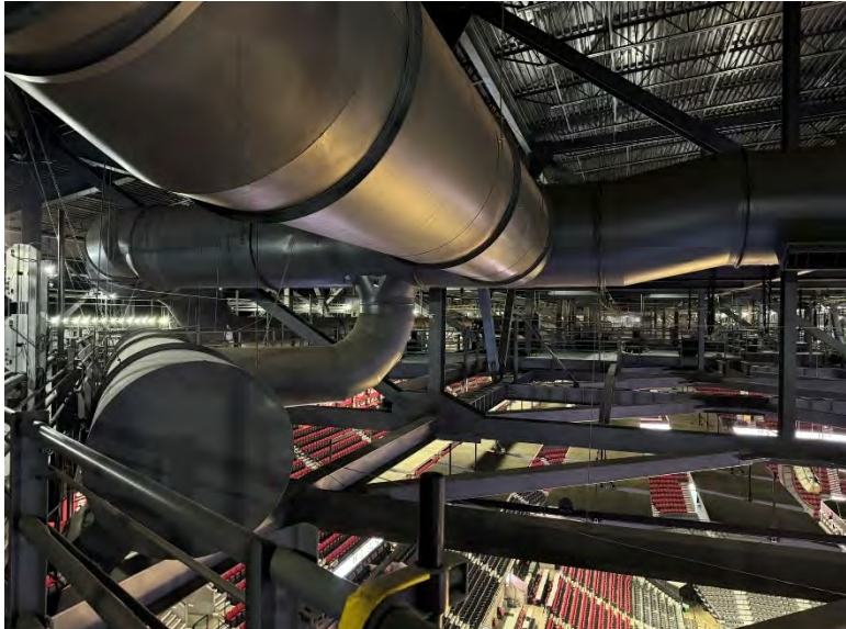
Arena air supply ductwork
