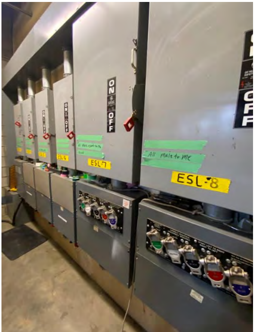
Northwest show power room
