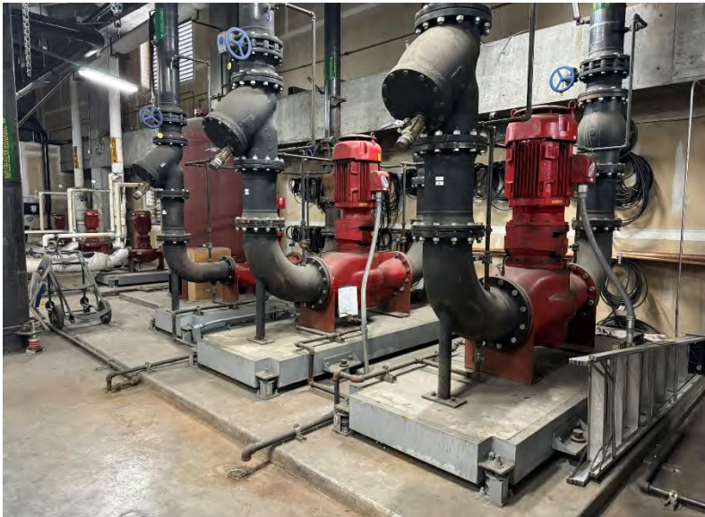
Condenser water pumps
