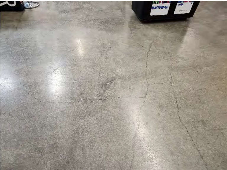
Preferred level (Section 209) concrete topping slab cracking
