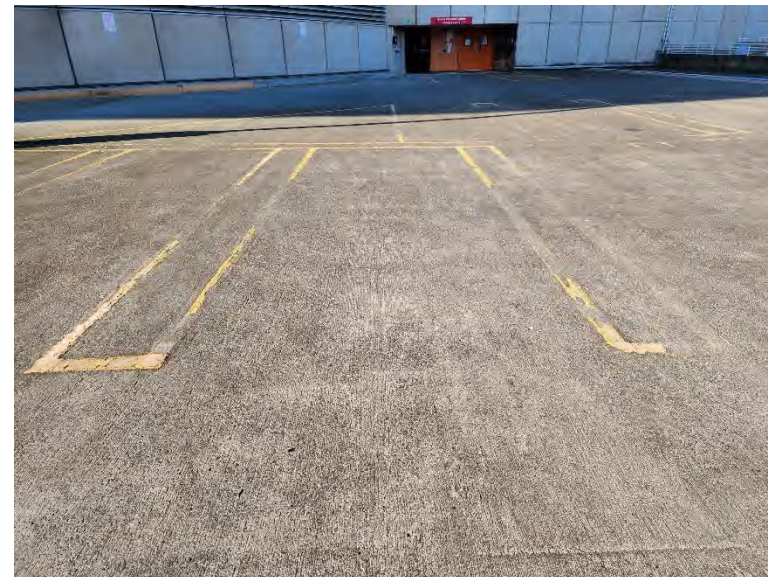
Level P7 faded parking stall striping
