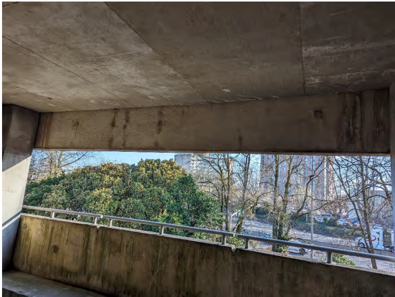
Level P6 efflorescence at perimeter façade panels below walls and curbs without cove sealant
