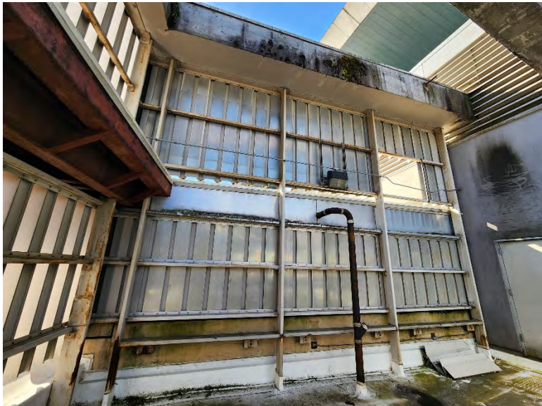
Mechanical level (Gridline R82-FF) corroded steel panels
