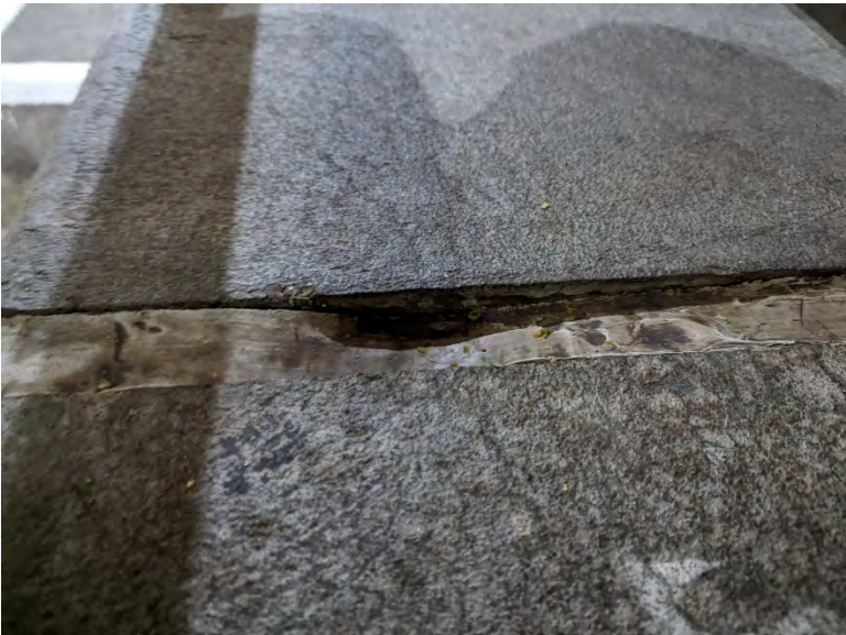
Seating bowl (Section 320) with locally failed joint sealant at seating row
