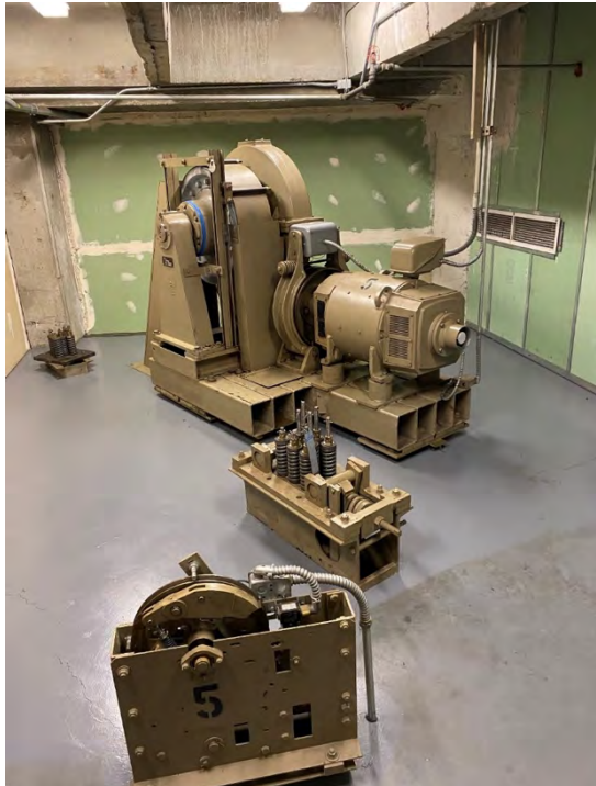
The machine room is clean and well organized
