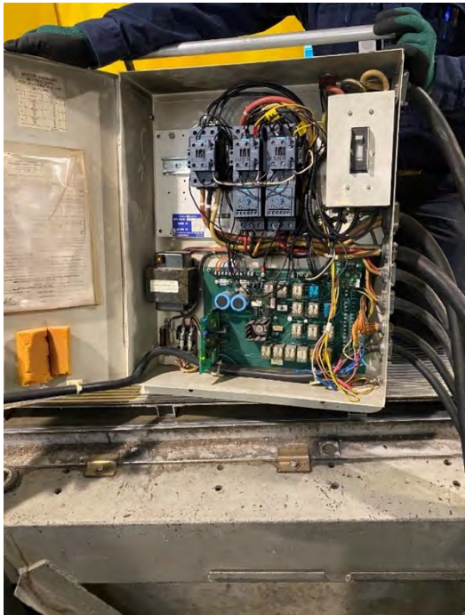
Typical controller in all escalators
