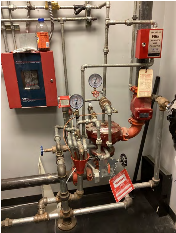
Pre-action deluge sprinkler valve serving the broadcasting area
