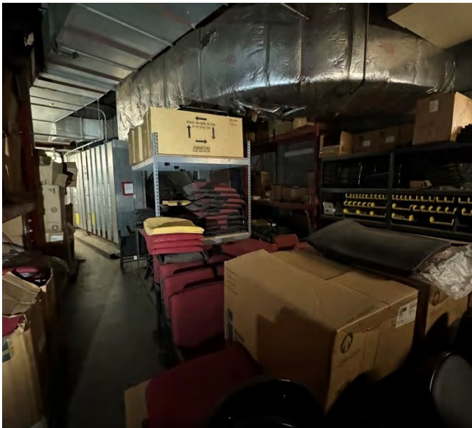
Obstructed air handling unit
