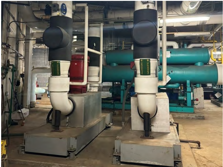
Chilled water secondary pumps
