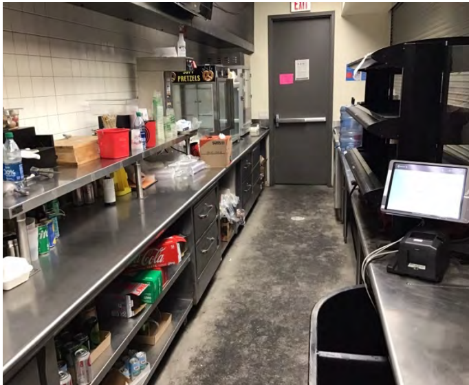
Concession flooring requiring power wash
