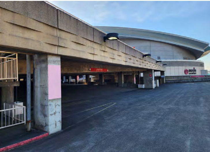
Dirt accumulation on precast panels
