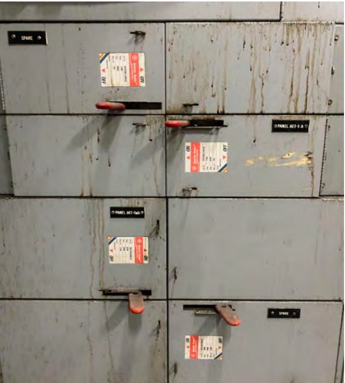
Liquid residue on motor control centers (MCC)
