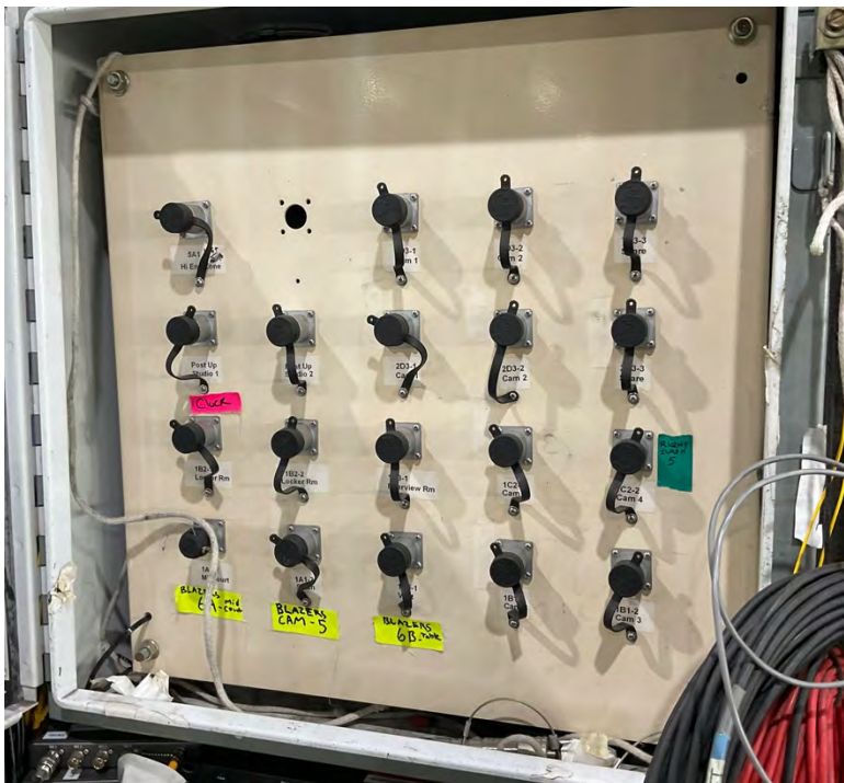
Broadcast truck dock cabling connections
