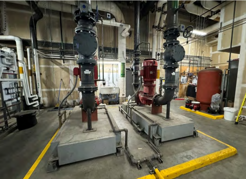
Heat recovery water distribution pumps
