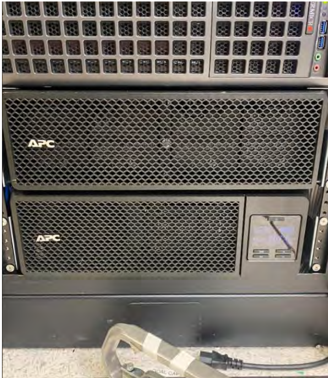
Rack UPS's serving server room
