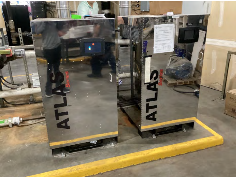
Domestic hot water boilers on club level
